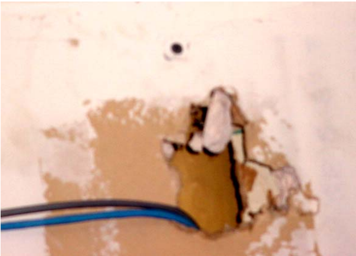
Open Utility Hole above Ceiling Plenum in Reception Area
