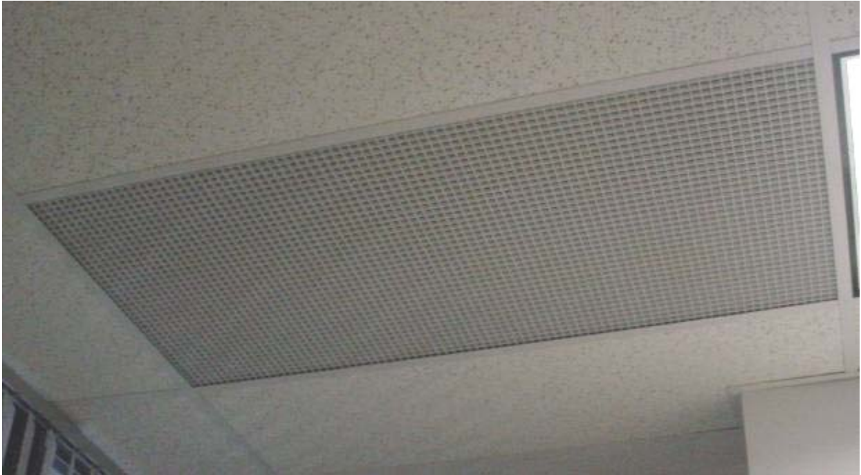
Return Grate to Ceiling Plenum
