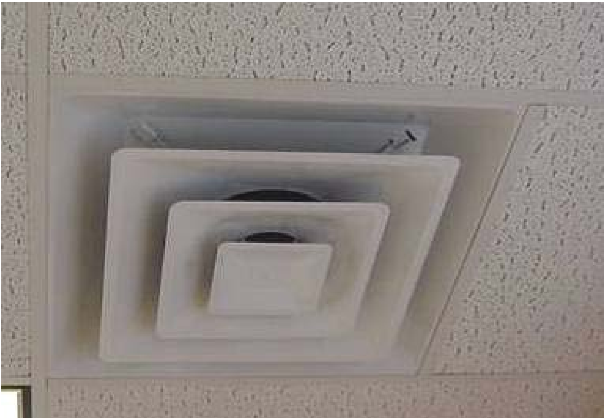
Example of Ceiling-Mounted Supply Air Diffuser
