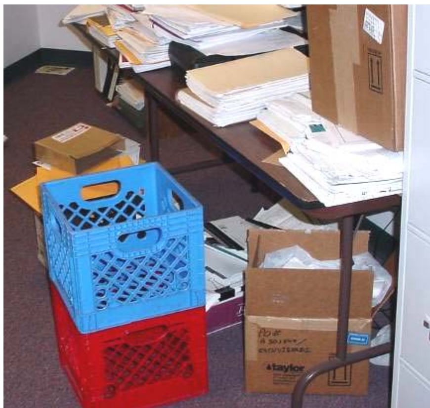
Porous Materials (Boxes, Papers) Stored in Area of Historic Water Damage
