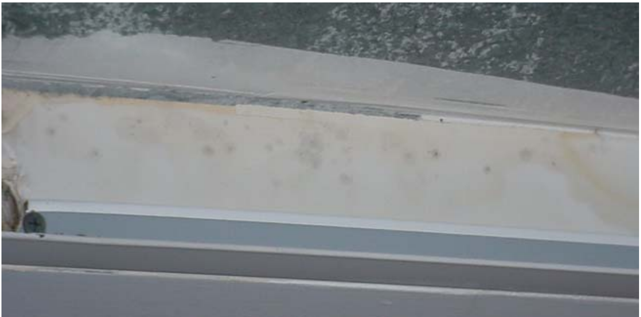
Visible Mold Growth (as Indicted by Dark Stains) on GW above Water Damaged Ceiling Tiles in Reception Area Lobby, Shown in Preceding Picture
