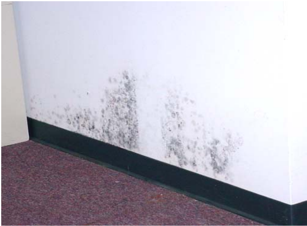
Visible Mold Growth (as Indicted by Dark Stains) on GW behind File Cabinets in Central Inspector's Area
