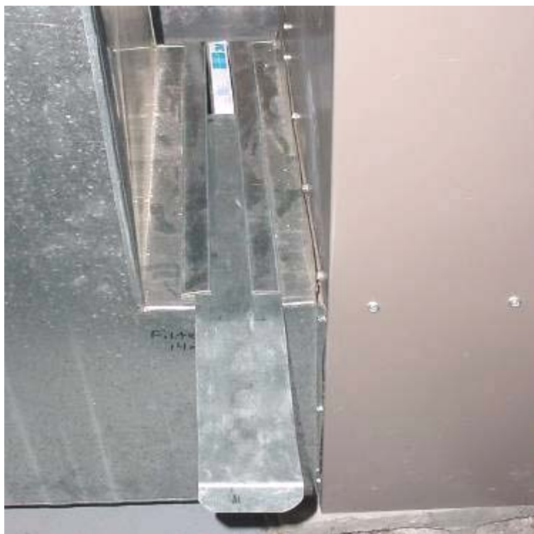
Example of Heat Pump Filter Slot Sealed With Sheet Metal Tab
