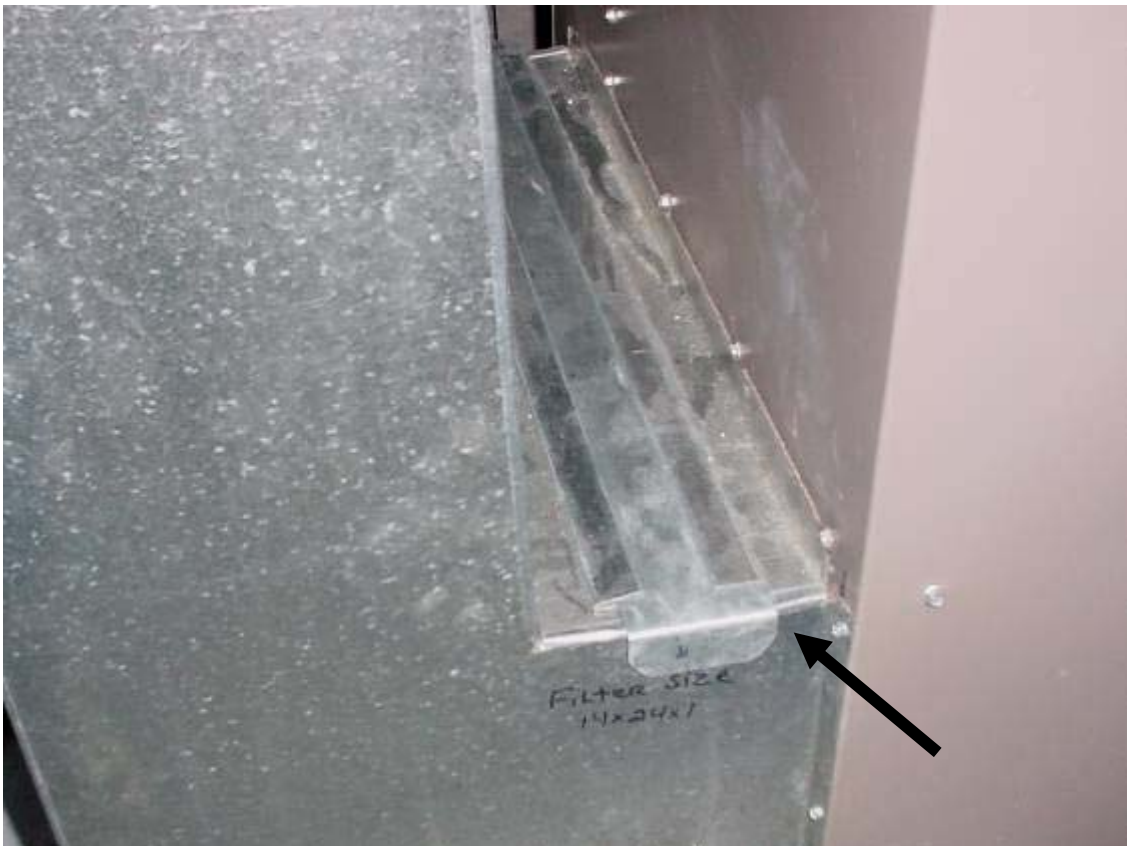
Example of Heat Pump Filter Slot Sealed With Sheet Metal Tab
