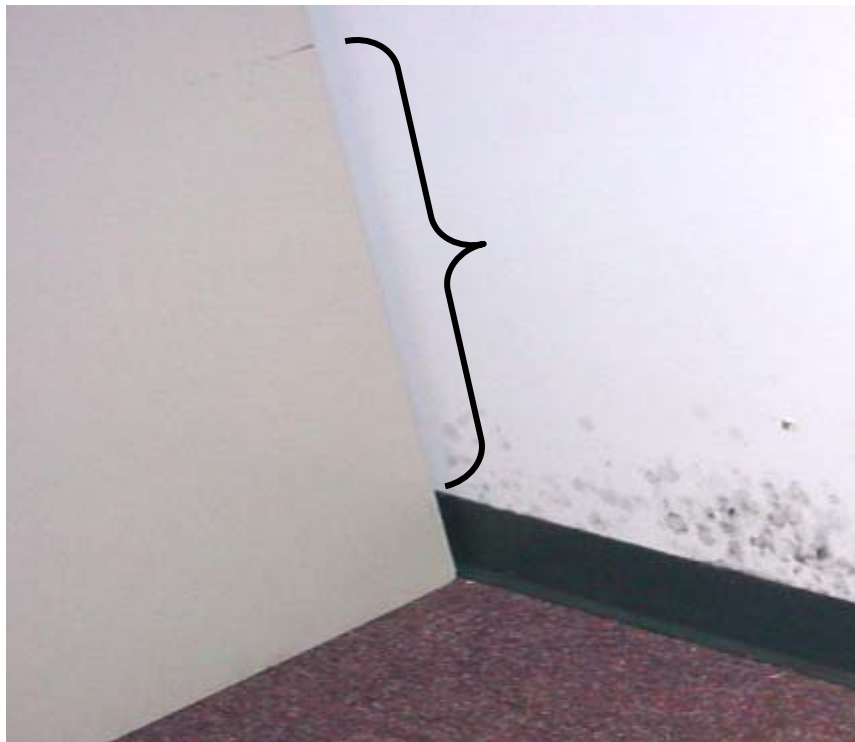
Close-Up of File Cabinets Directly against Wall in Central Inspector's Area
