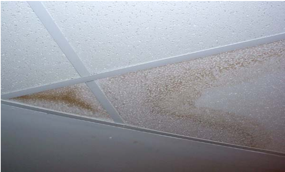
Water Damaged Ceiling Tiles in Reception Area Lobby
