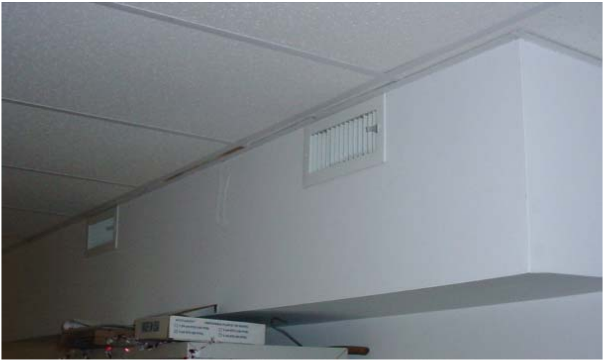
Ducted Supply Diffusers
