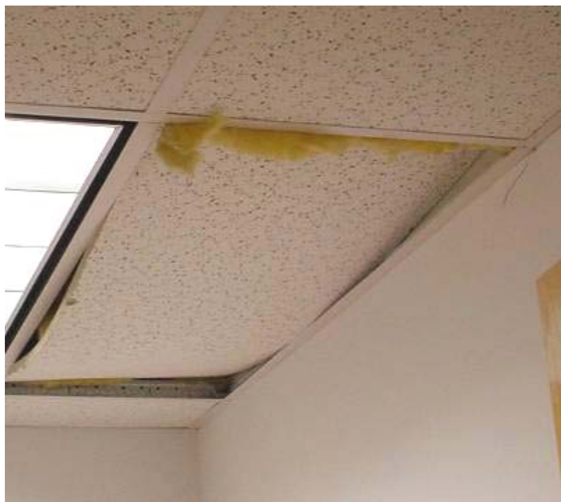
Exposed Fiberglass Insulation in Storage Room
