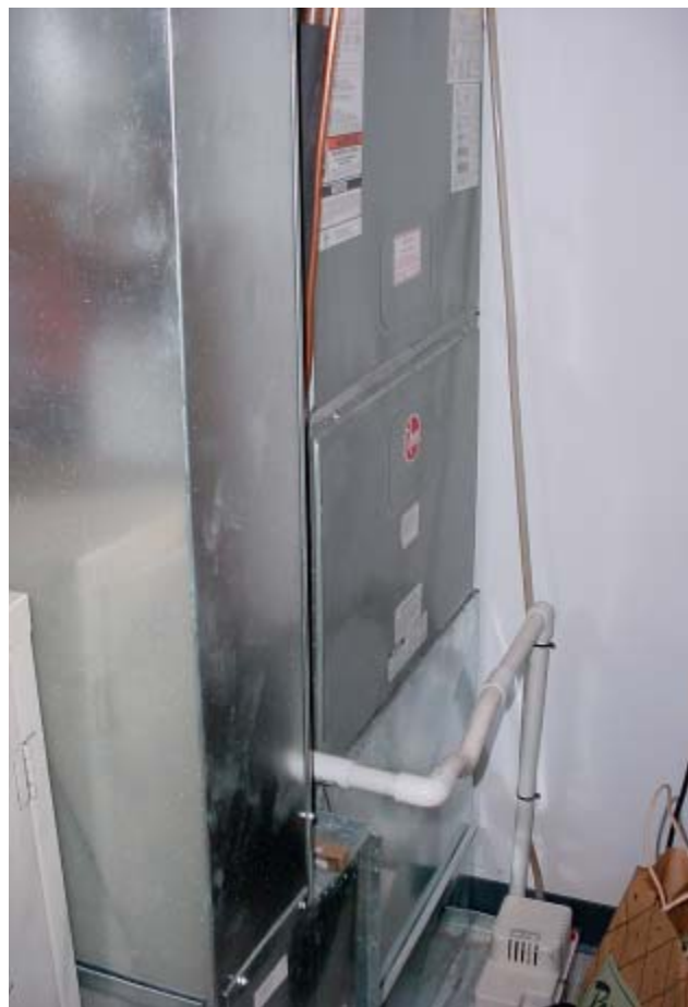
One of Two Heat Pumps Located in Mechanical Closets
