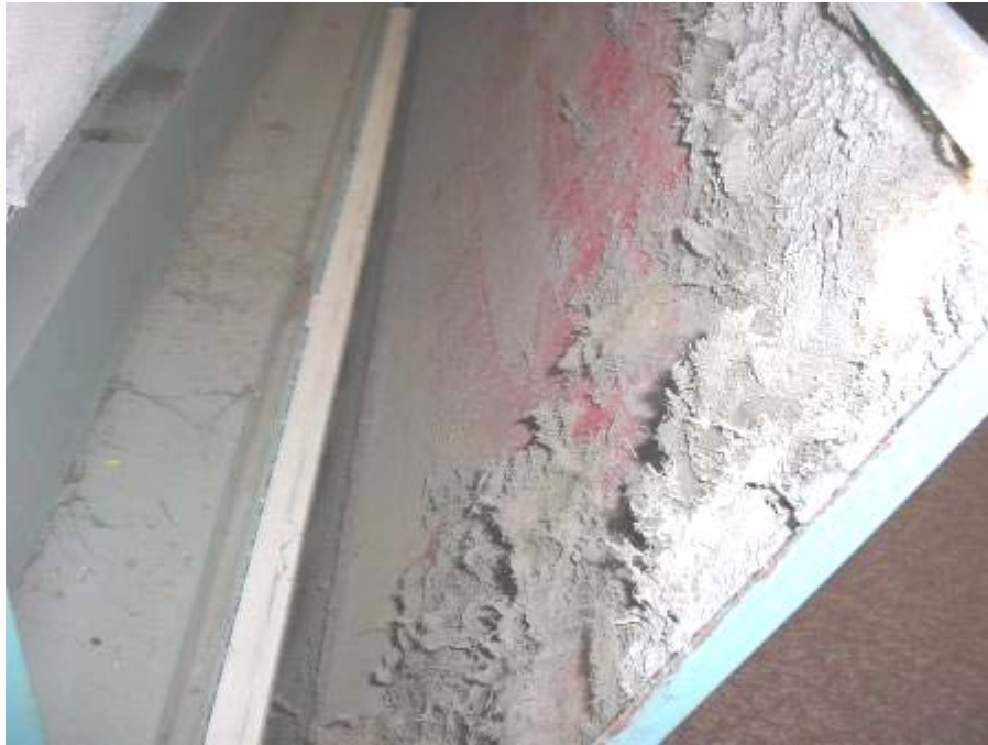
Disintegrating Fiberglass Insulation in Univent
