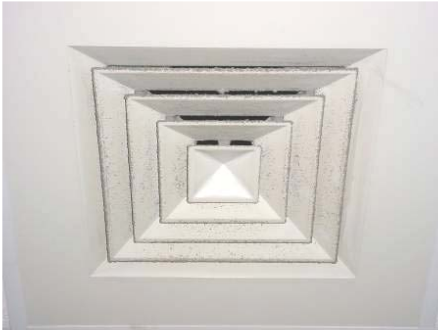
Exhaust Vent with Dirt and Dust
