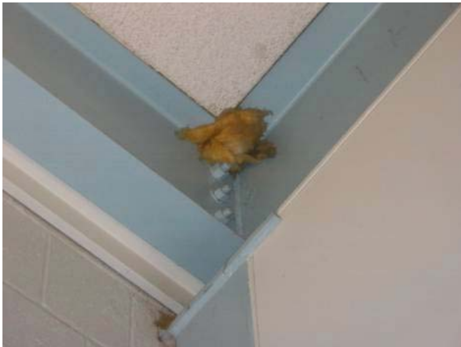
Exposed Fiberglass Insulation
