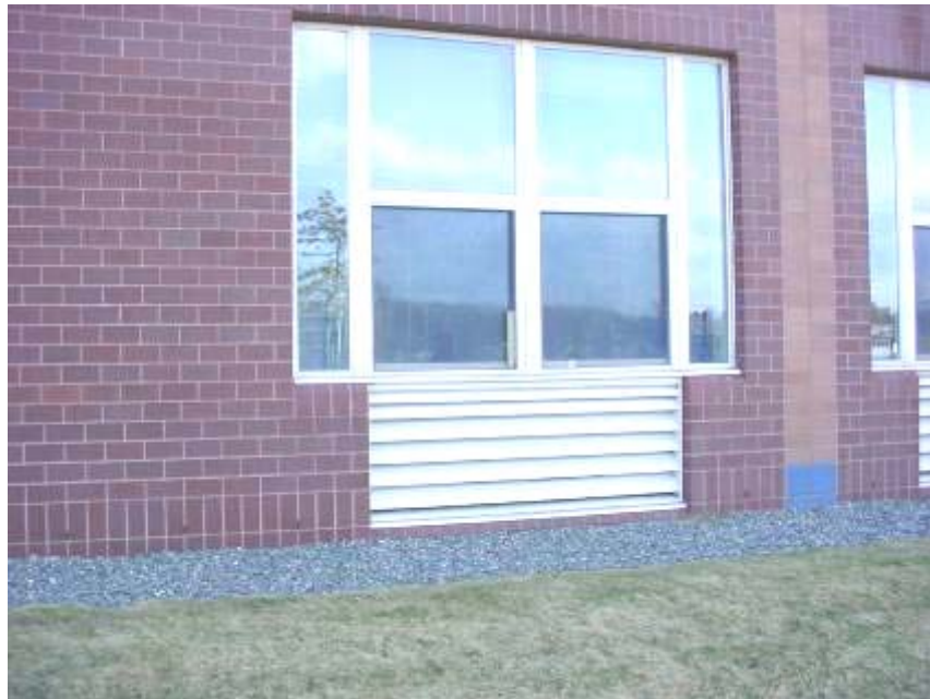
Fresh Air Intake
