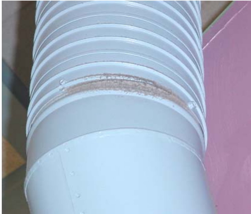
Breach in Exhaust Duct, Note Dust/Debris Accumulation
