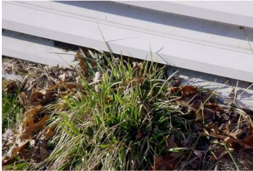
Plants/Leaves/Debris in/near Univent Air Intake
