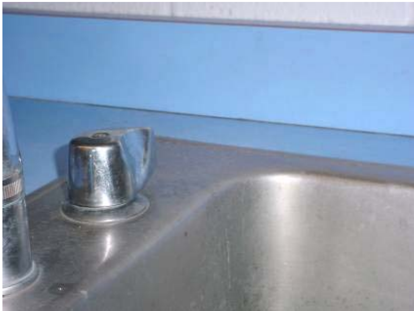
Open Seam between Sink Countertop and Backsplash
