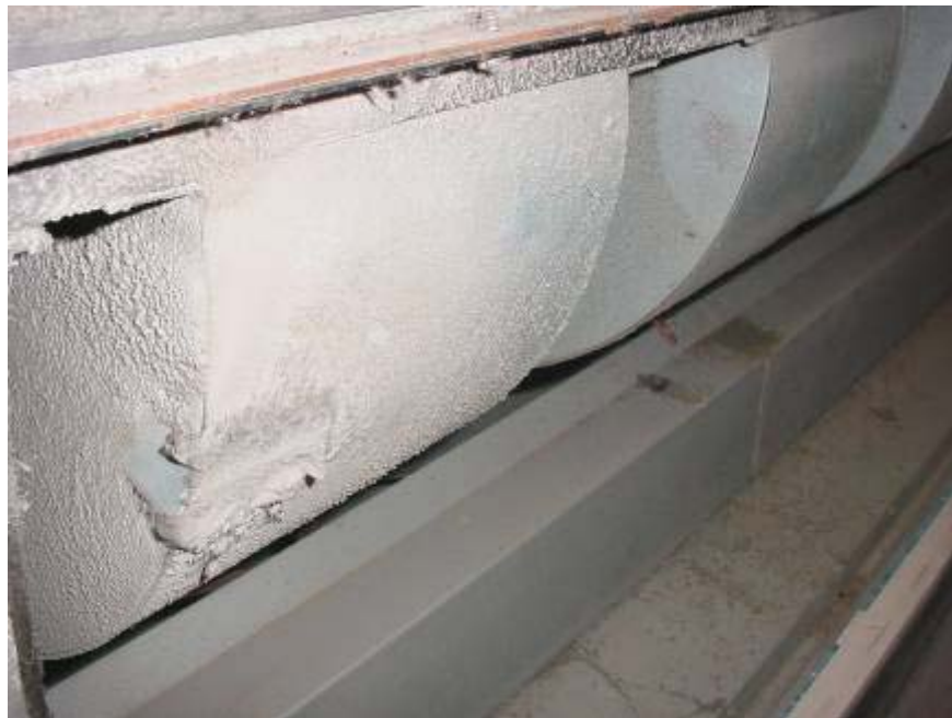
Dirt, Dust, Debris Buildup in Univent
