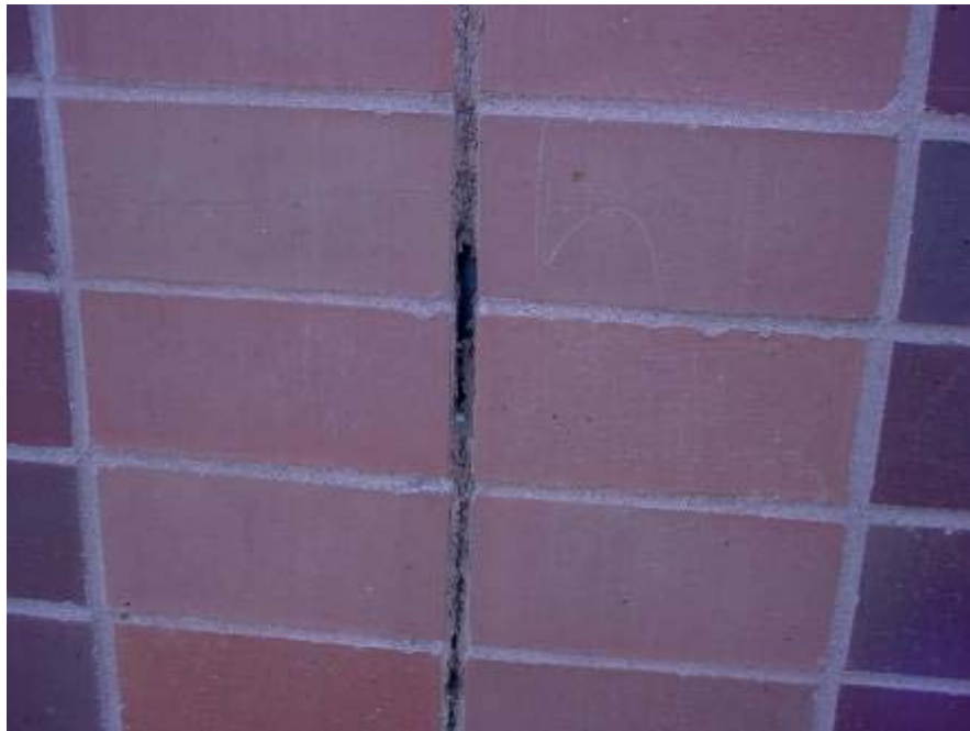
Expansion Joint with Missing/Damaged Sealant
