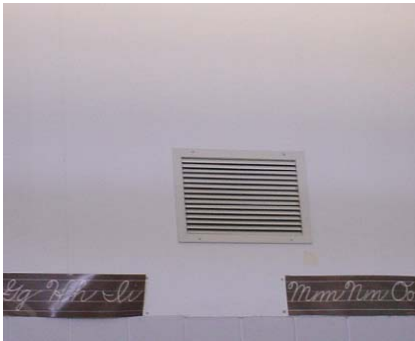
Wall-Mounted Exhaust Vent
