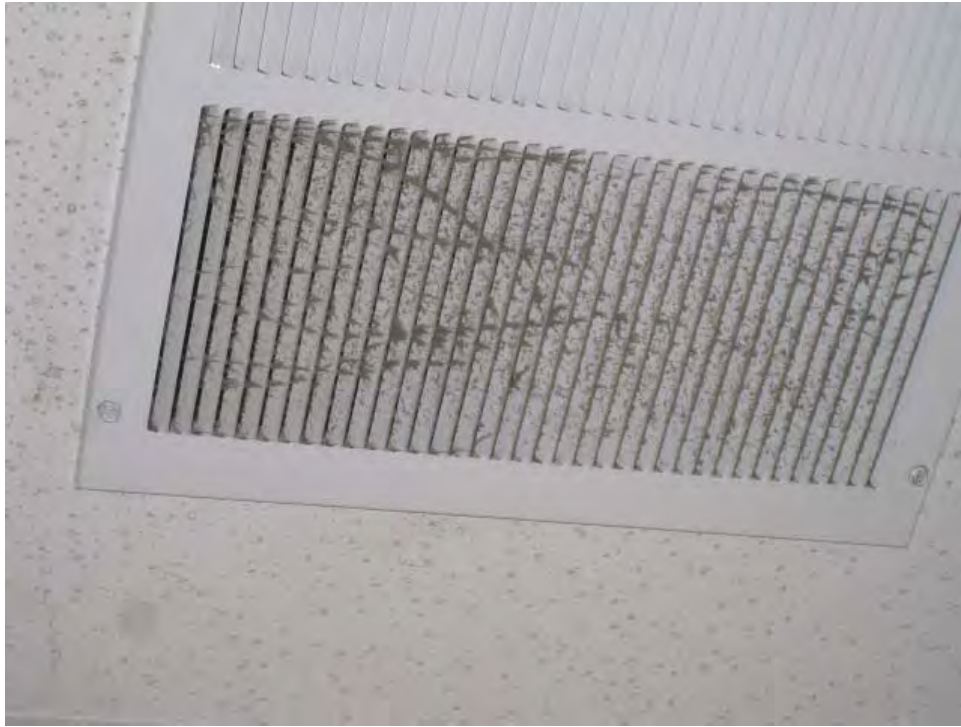
Example of Dirty Exhaust Vent
