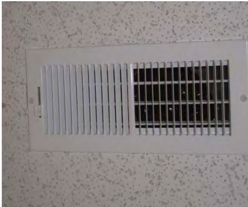
Typical Fresh Air Supply Vent
