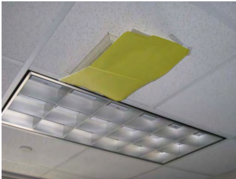
Supply Vent Blocked with Cardboard
