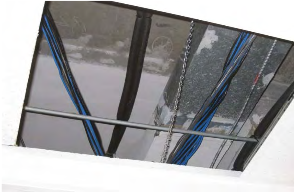
Missing Ceiling Tile
