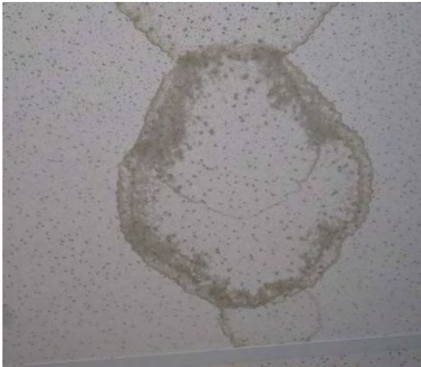
Water-damaged Ceiling Tile
