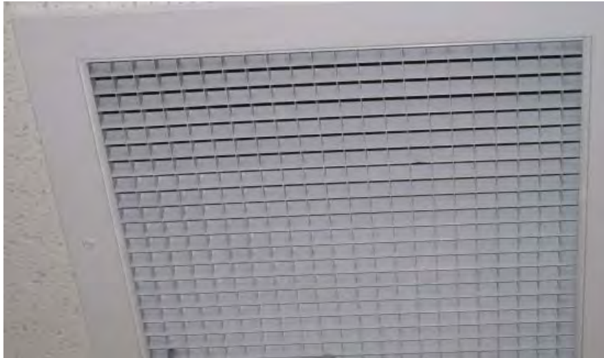
Ceiling Exhaust Vent
