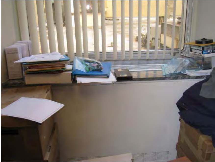
Obstructed Fan Coil Unit
