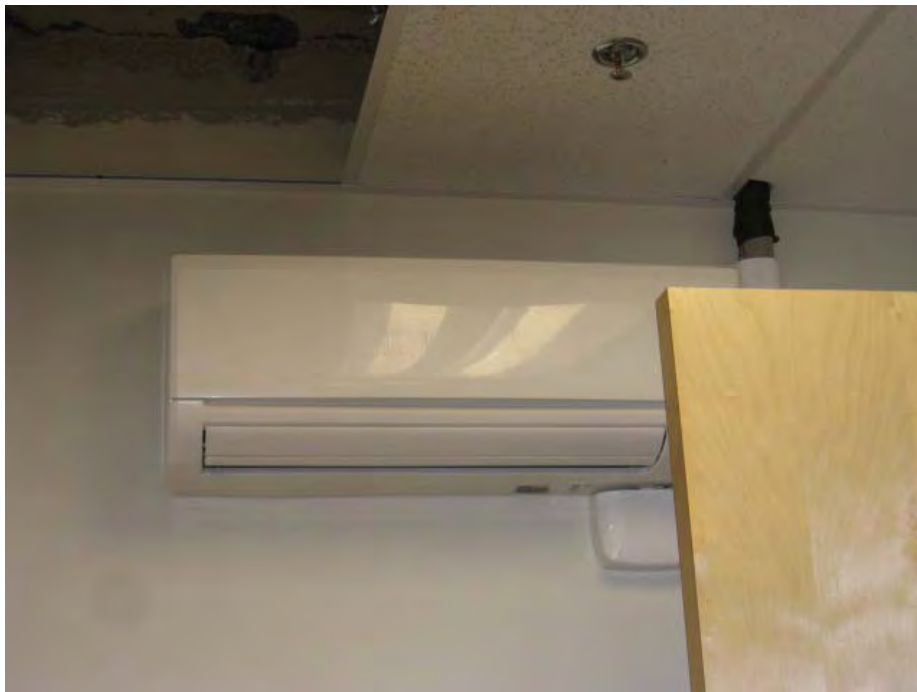
Typical Wall-Mounted Fan Coil Unit
