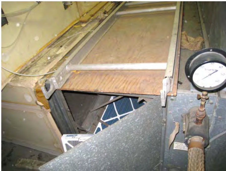
AHU with access doors open
