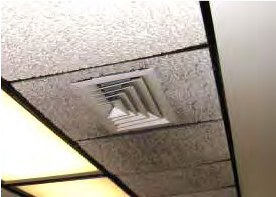
Soiling of ceiling tiles around fresh air supply diffuser
