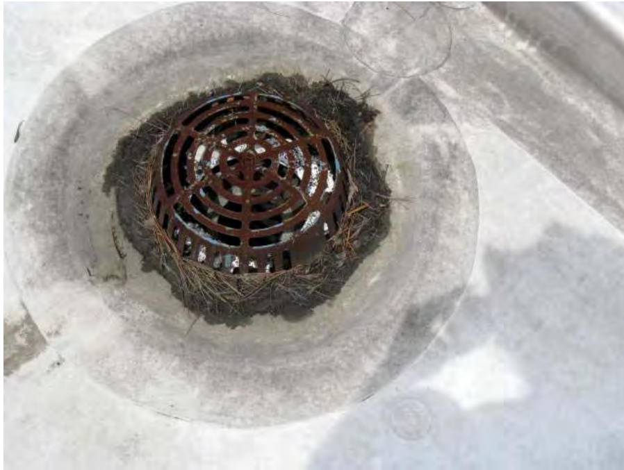
Roof drain installed at a point higher than level of roof
