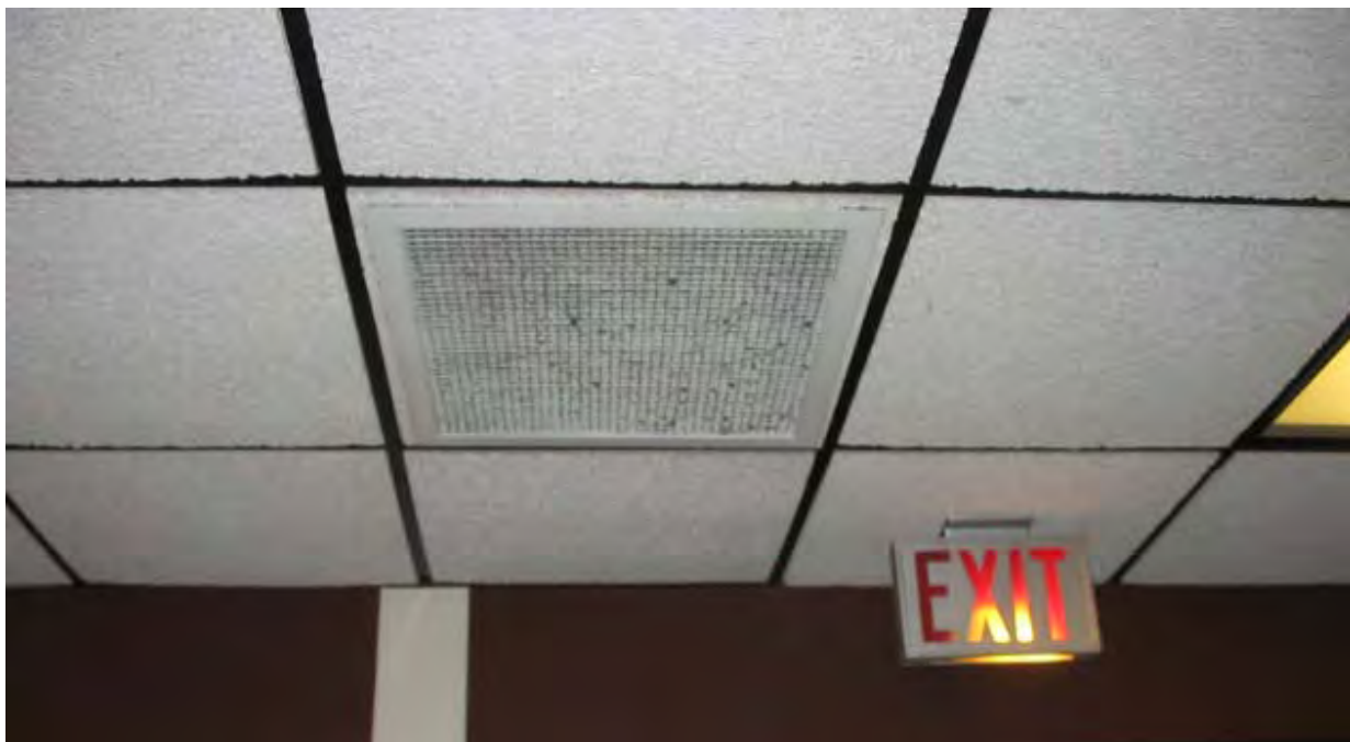
Bowing ceiling tiles
