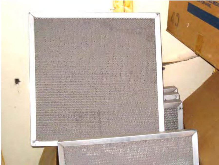
Wire mesh filters, note occlusion with dust/debris
