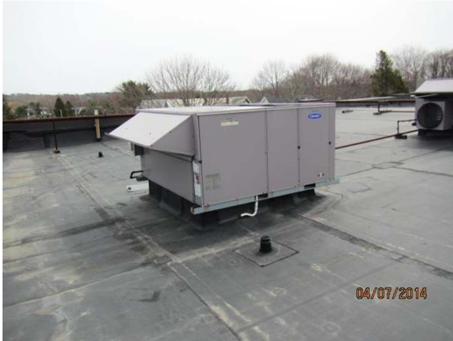
Air handling unit (AHU) on the roof
