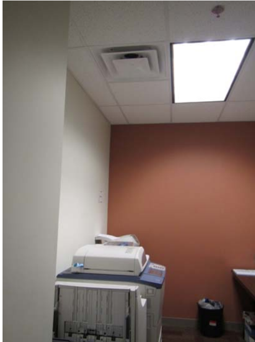
Photocopier directly below supply vent
