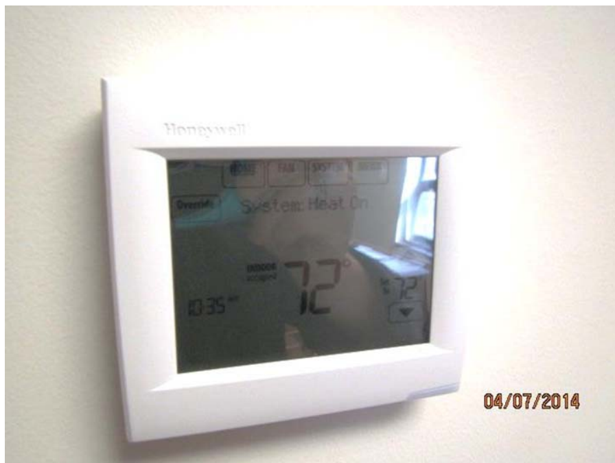
Thermostat in the office
