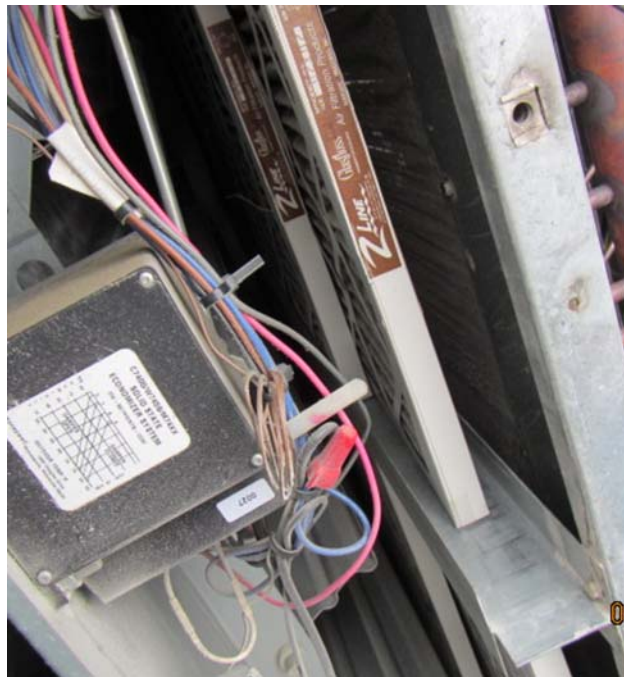
Opened rooftop AHU showing wrong-sized filter
