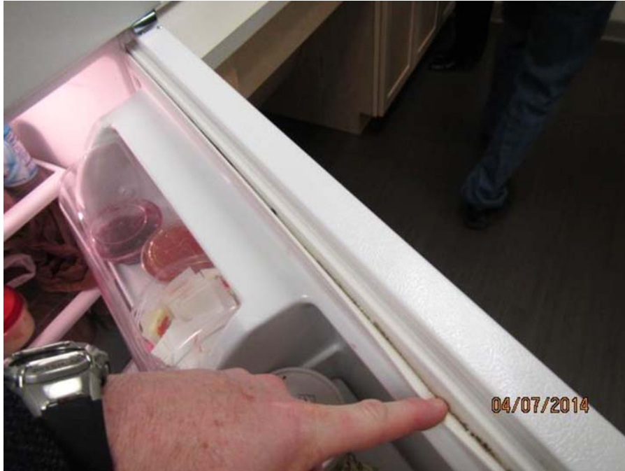
Mold-colonization (dark staining) on refrigerator gasket
