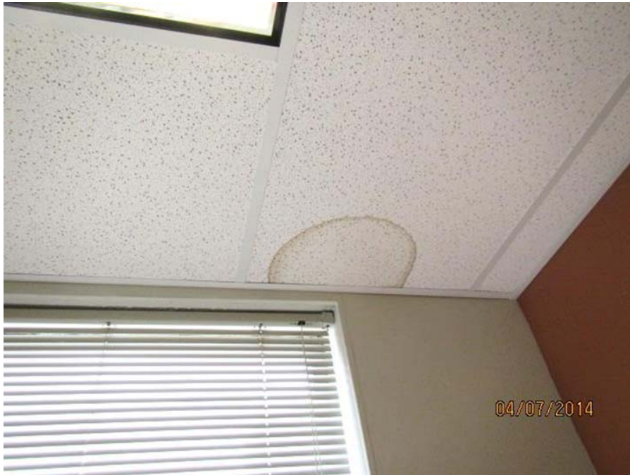
Water-damaged ceiling tile
