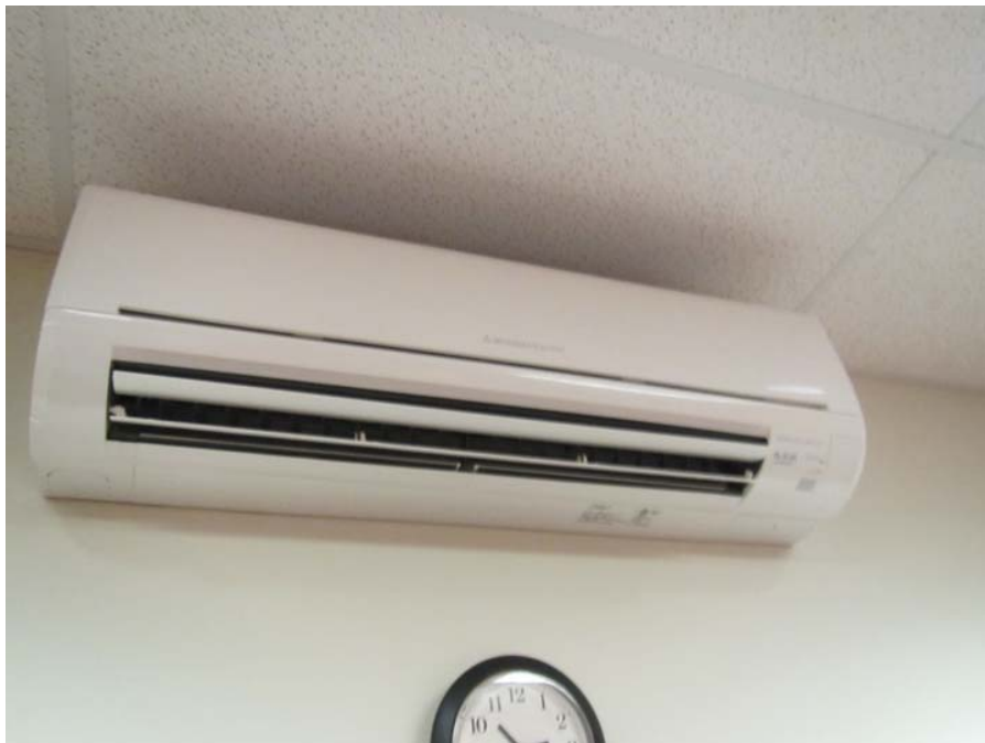
Ductless air conditioning unit
