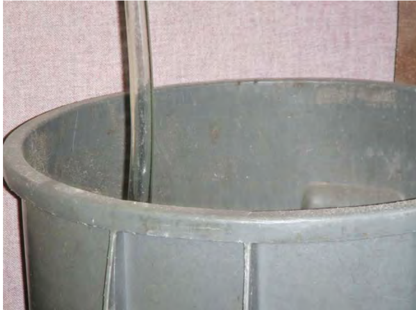
Drainage hose terminating into a barrel in room 286
