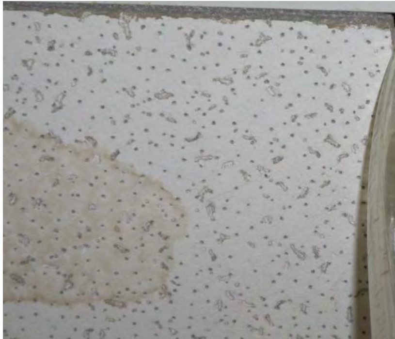
Water-damaged ceiling tile above Room 286
