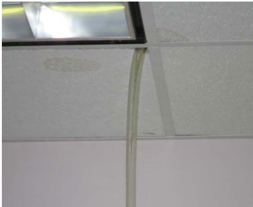
Drainage hose extending from ceiling plenum above room 286
