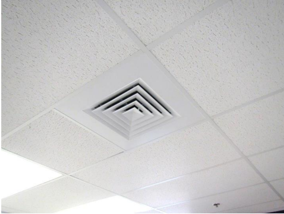
One type of supply vent in the DOR offices
