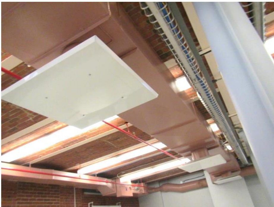
Supply vent in open areas of the DOR office
