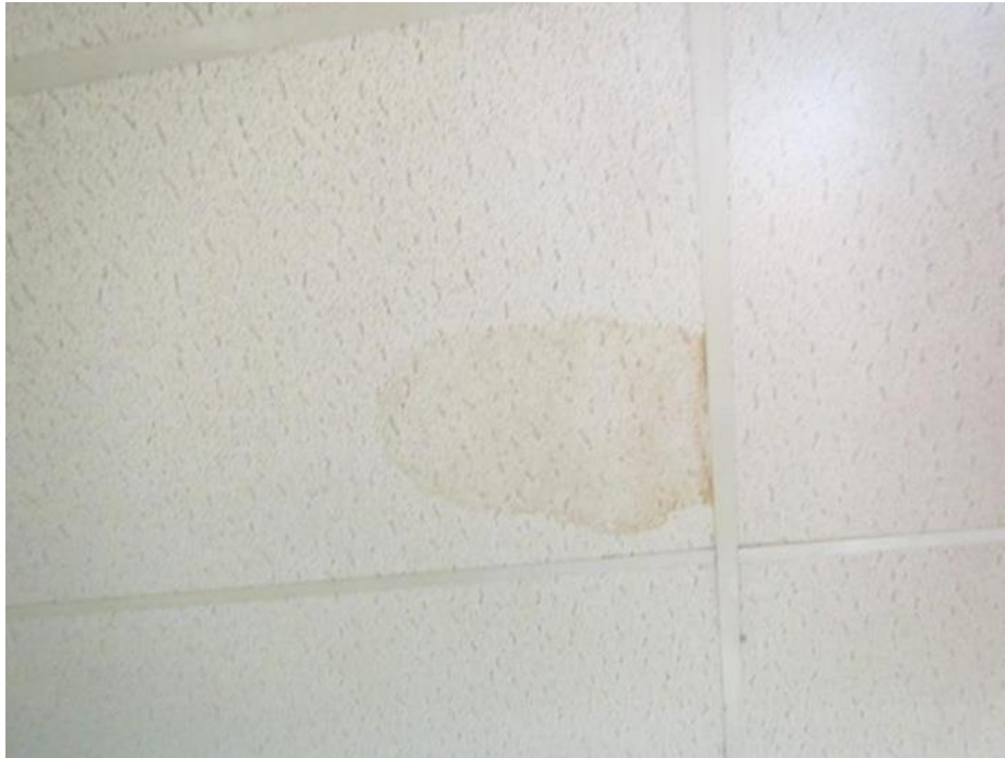
Water-damaged ceiling tile in men's restroom
