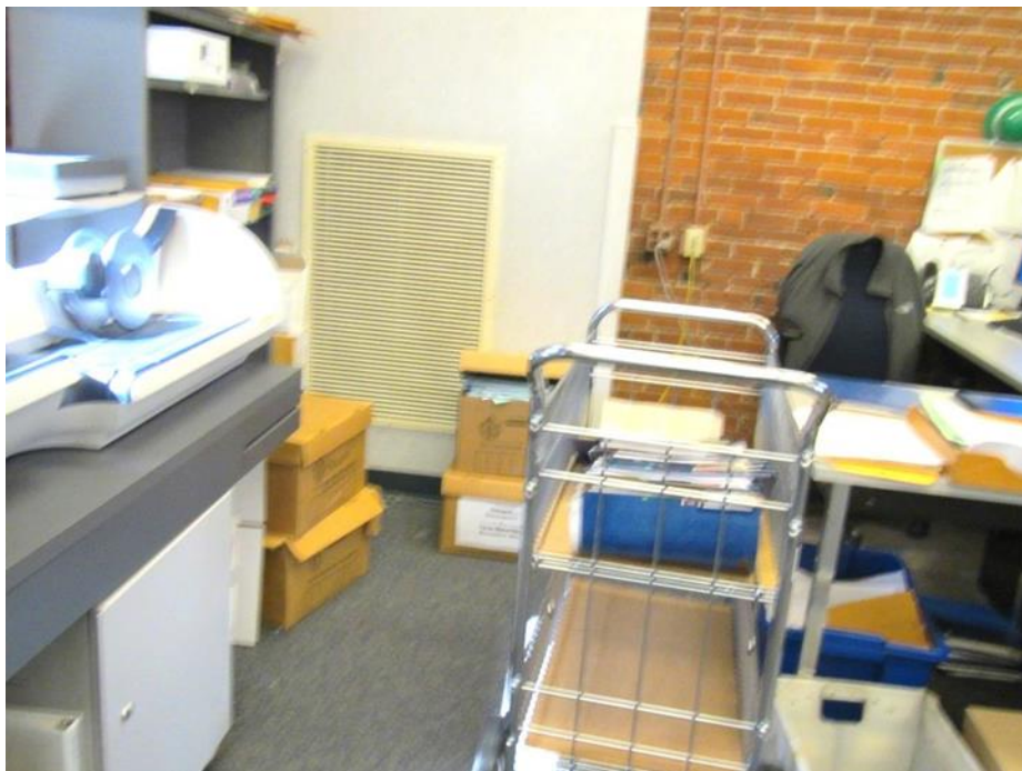
Wall-mounted exhaust vent
