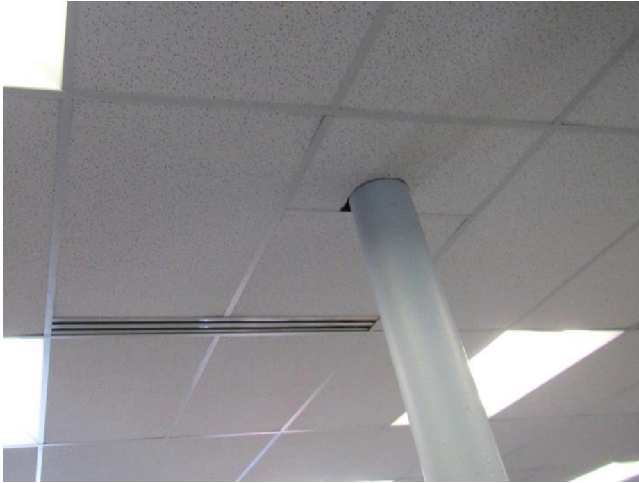
Slot-style supply vent
