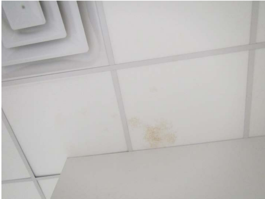
Water-damaged ceiling tile in conference/storeroom
