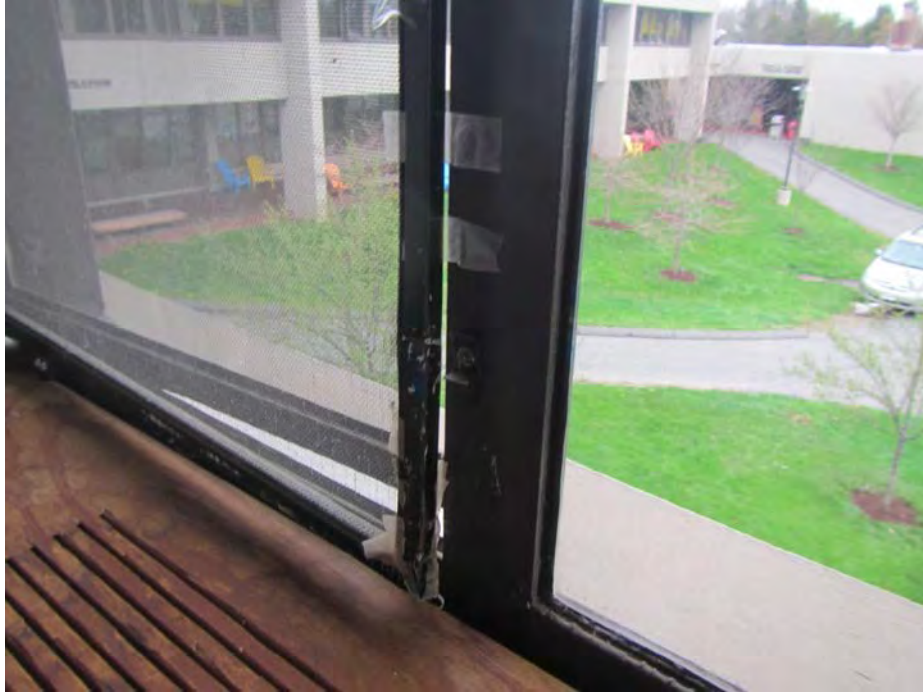
Screen not attached to window frame
