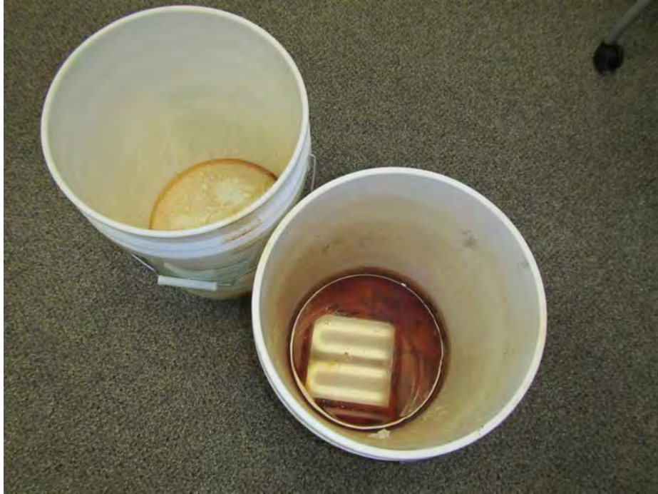
Buckets used in room K213 to catch active water leaks
