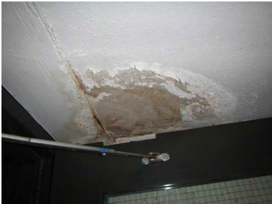
Water-damaged ceiling in K210 hallway
