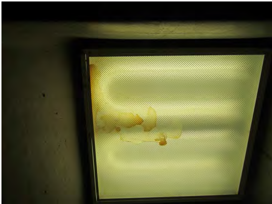
Active water leak above light fixture in room K213
