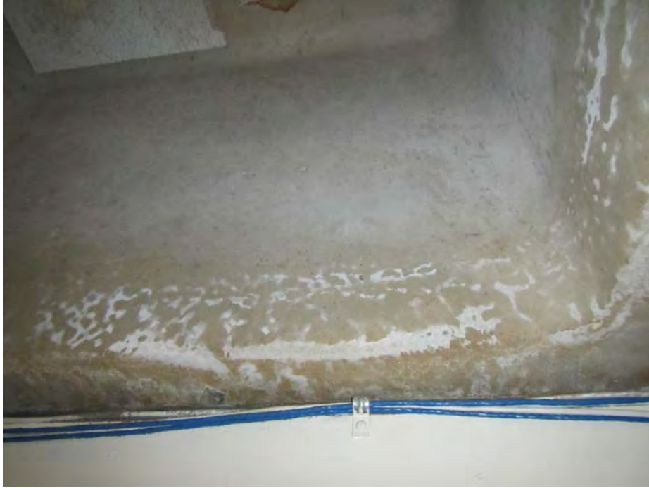
Efflorescence (white deposits) on concrete ceiling
