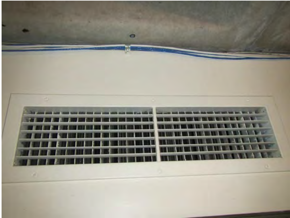
Supply air diffuser in Testing Room (K213)
