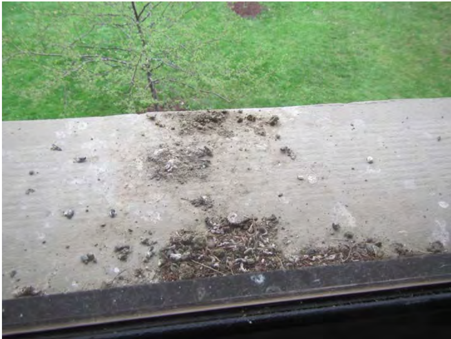
Bird waste and nesting debris outside of window in room K214A
