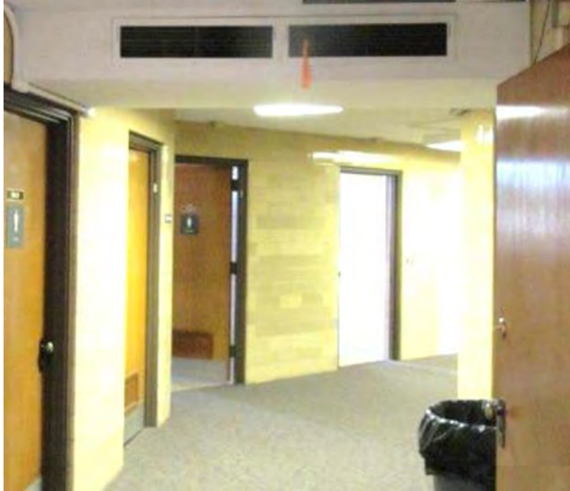
Hallway supply vents
