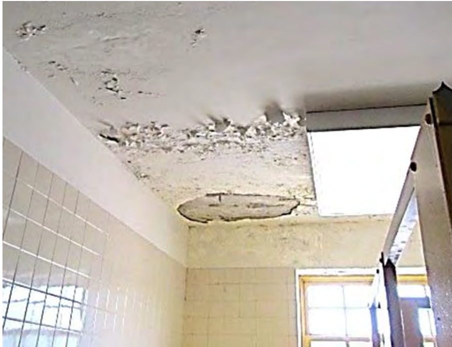
Severely water-damaged ceiling in 3 rd floor women's restroom
