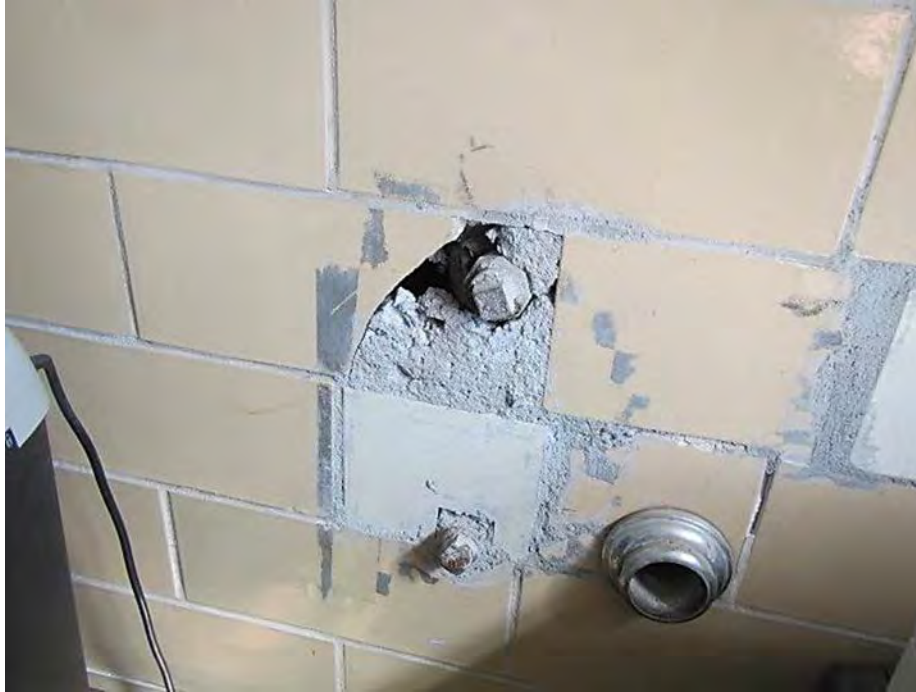
Hole in wall around utility pipe
