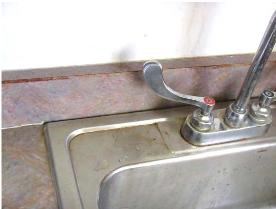
Loose/damaged backsplash kitchen 228
