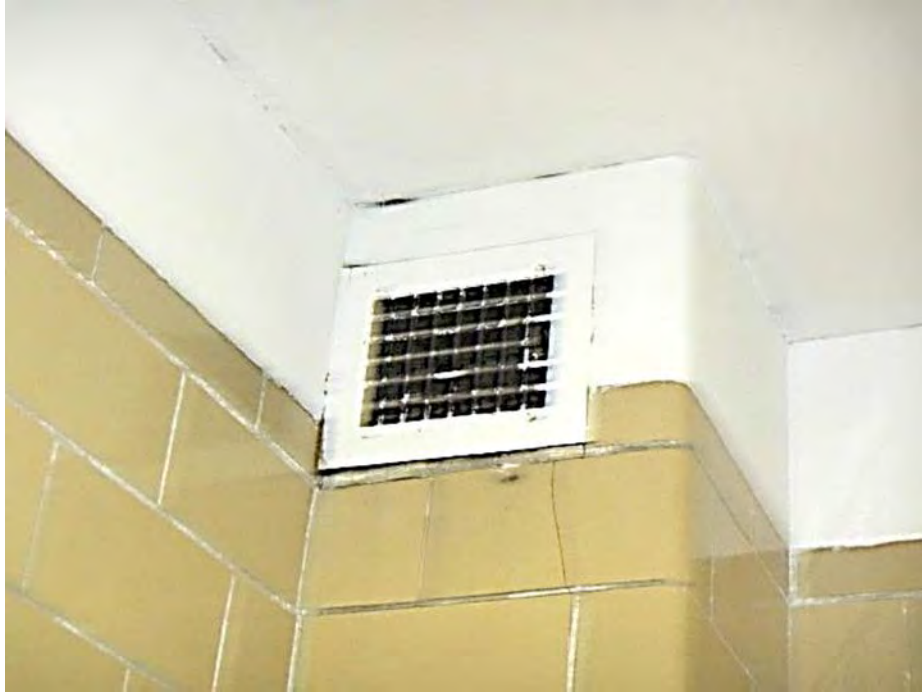
Wall-mounted exhaust vent, note dust/debris
