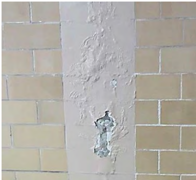
Peeling paint and efflorescence
