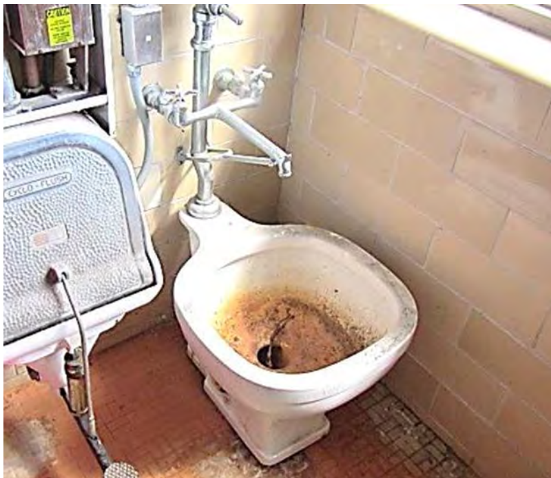
Abandoned toilet in room 256
