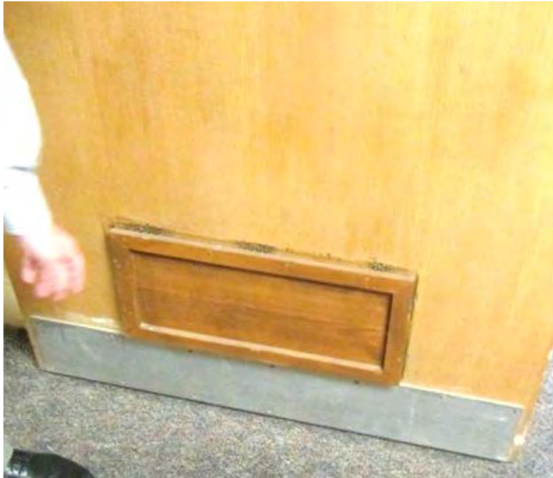
Sealed passive door vent
