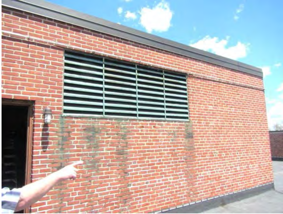
Fresh air intake for AHU
