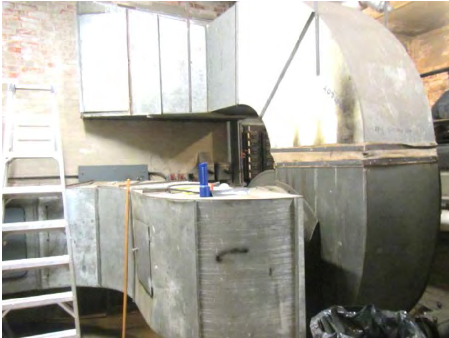
Air handling equipment in attic
