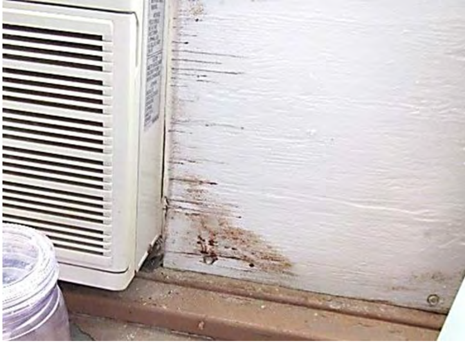
Water-damaged wood/possible mold growth on wood around AC room 456
