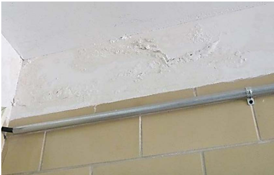
Peeling paint and efflorescence
