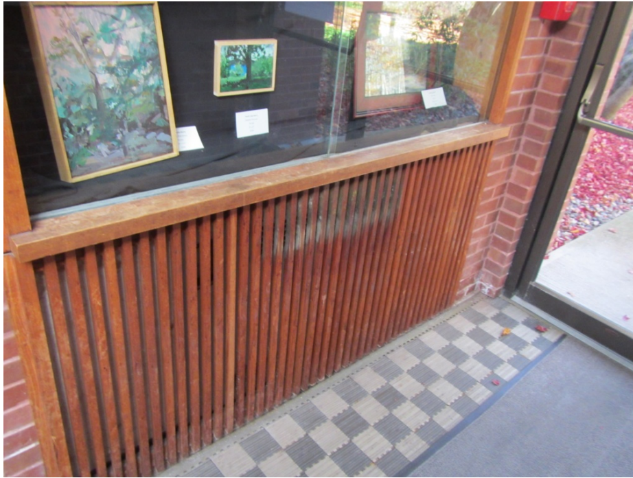
Mold-colonized wood on FCU cover in foyer
