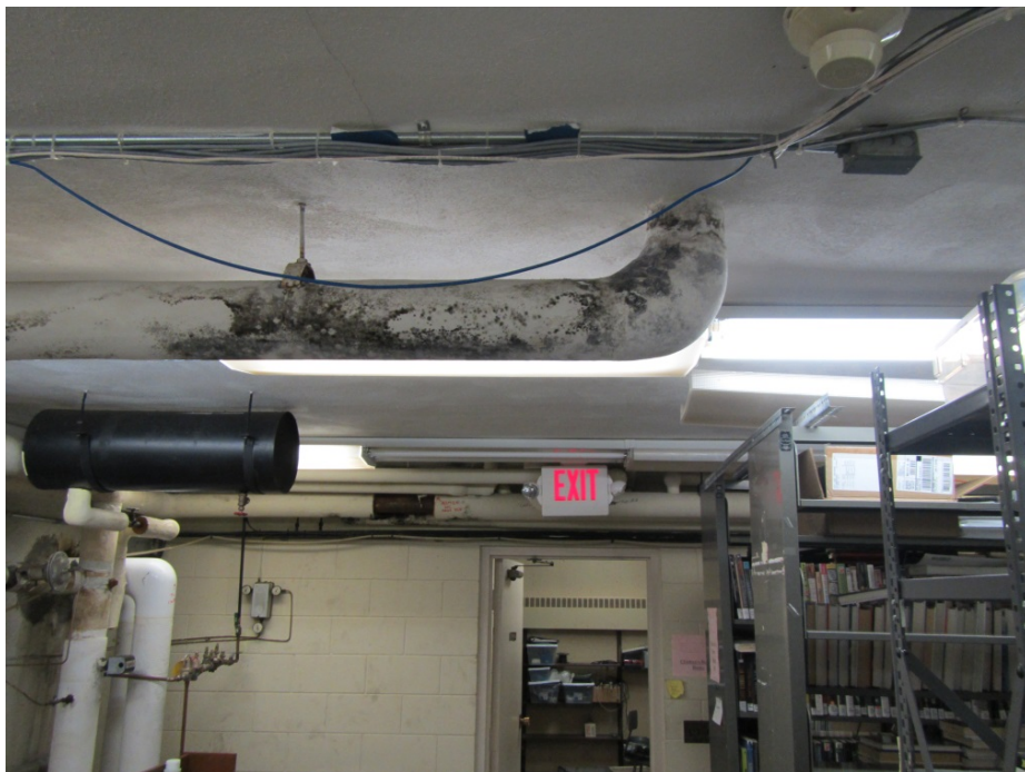
Mold-colonized pipe insulation in basement area
