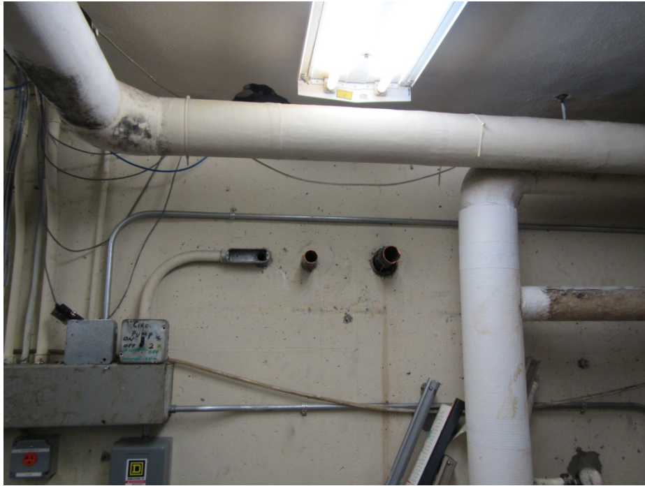
Open abandoned pipe/conduit in the basement area
