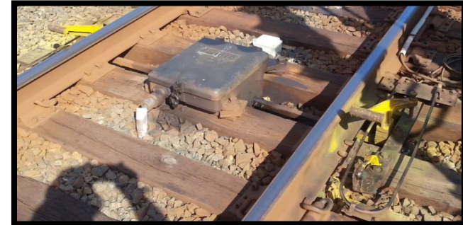
Installed Mechanical Trip Stop
