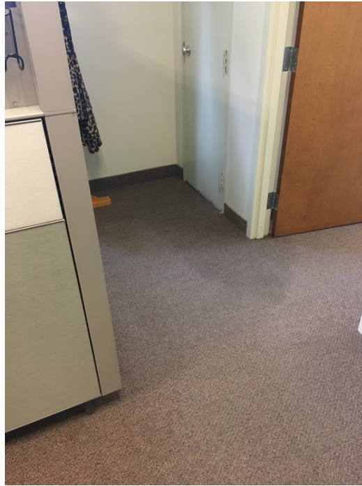
Moistened carpet outside utility closet
