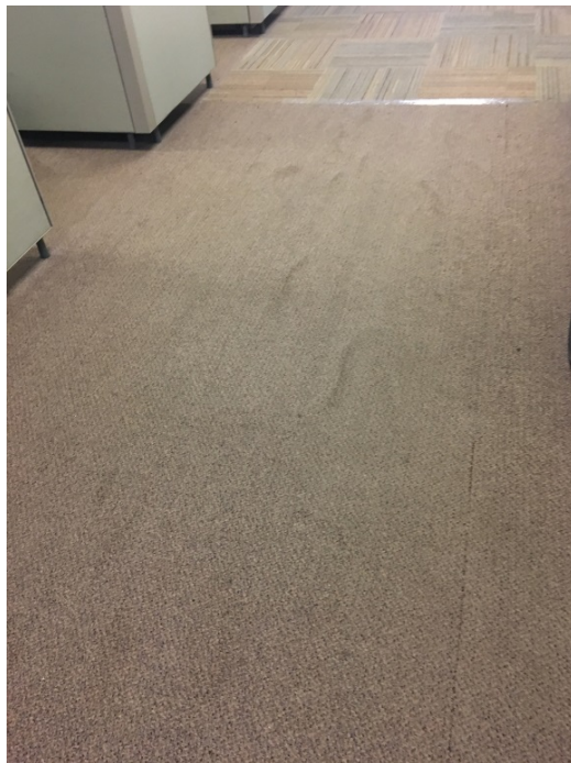
Rippled carpet, indicating water exposure
