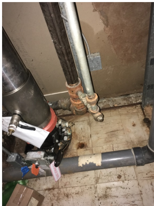
Floor of water-damaged utility closet
