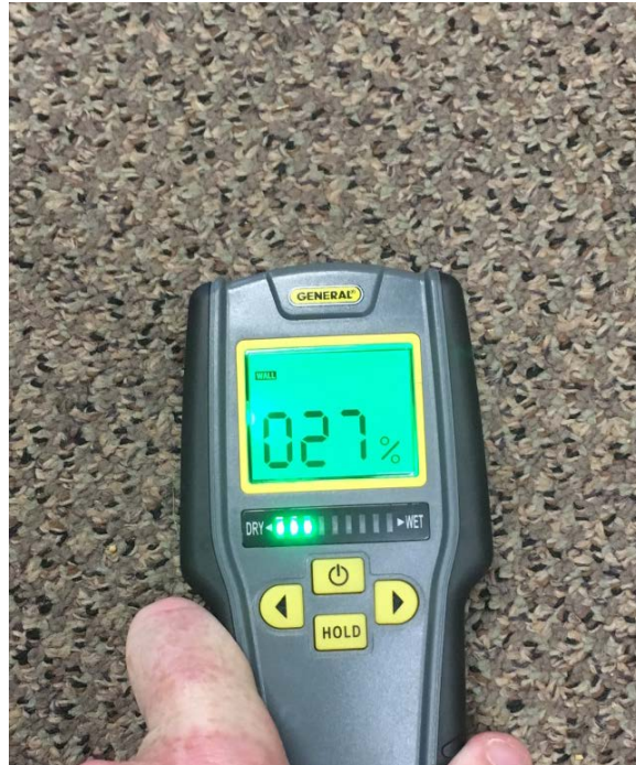
Moisture meter indicating moisture in carpet.
