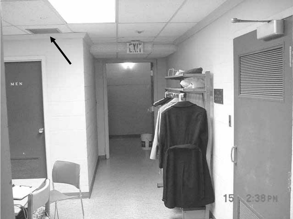
Ceiling-Mounted Exhaust Vent in Basement Breakroom
