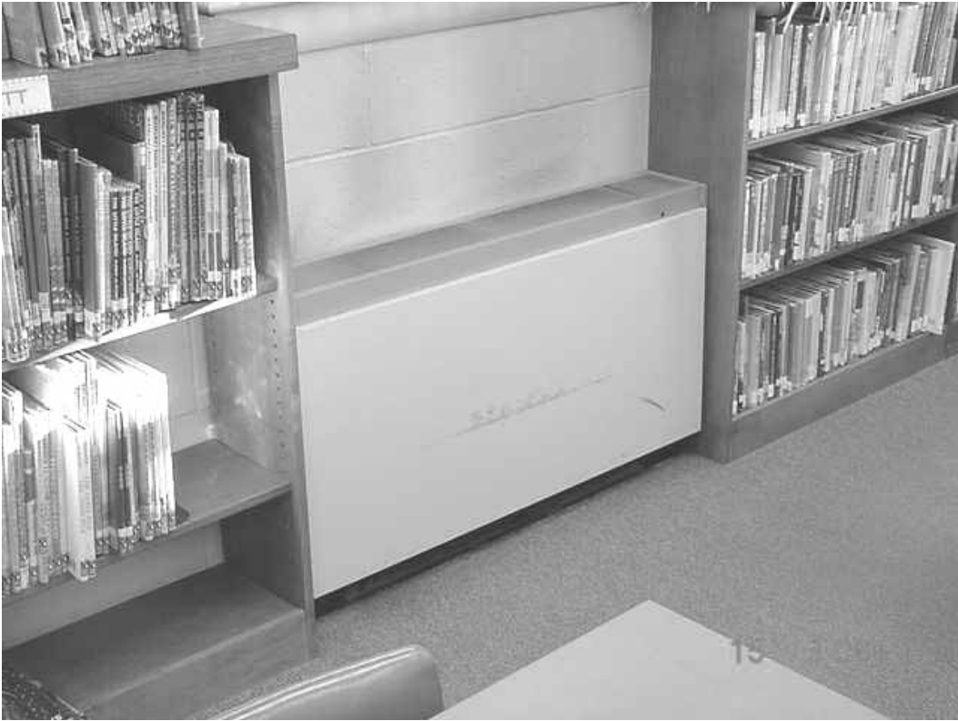
Example of Unit Ventilator on Main Floor
