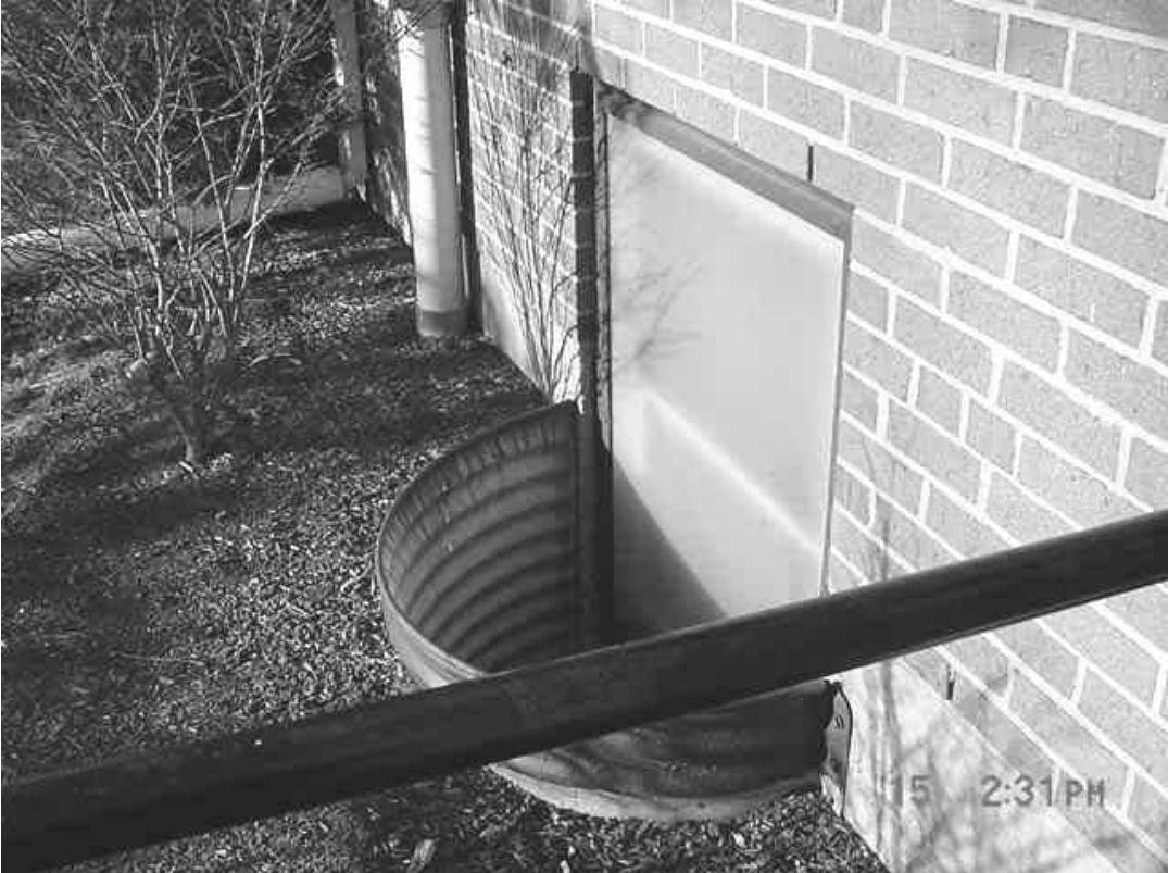
Basement Window Sealed With Plexi-Glass
