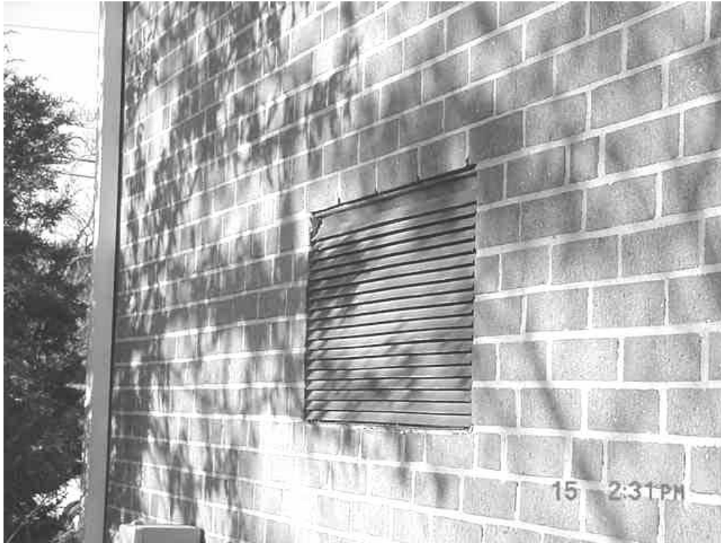
Univent Fresh Air Intake
