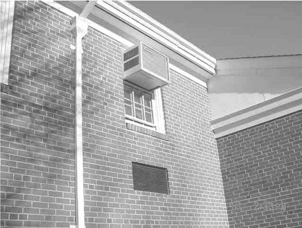
Portable Air Conditioning Unit Installed in Window
