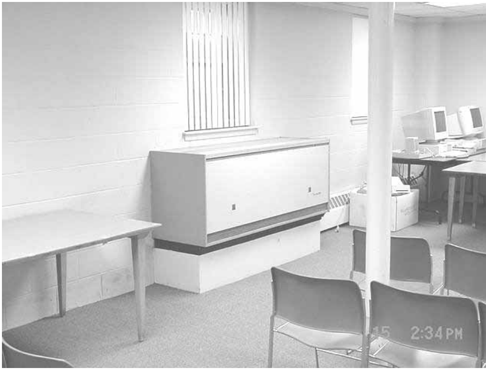
One of Two Basement Unit Ventilators
