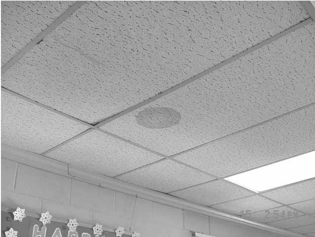
Water Damaged Ceiling Tile
