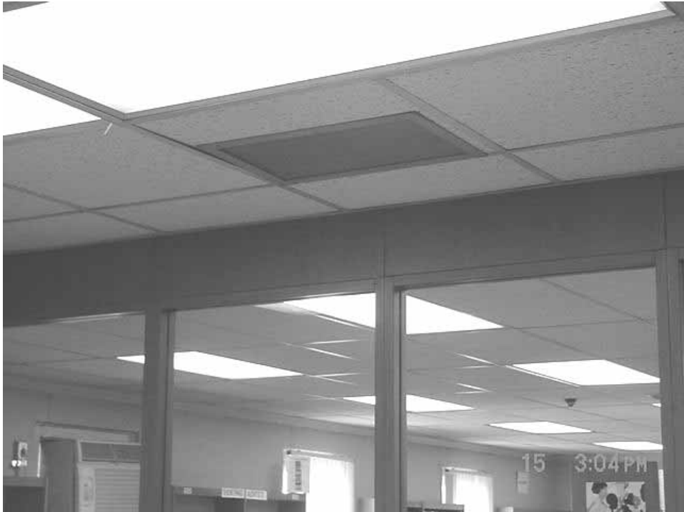
Ceiling-Mounted Exhaust Vent in Main Office
