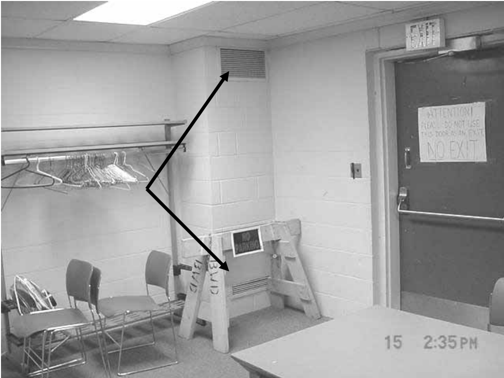
Wall-Mounted Exhaust Vents in Basement Auditorium
