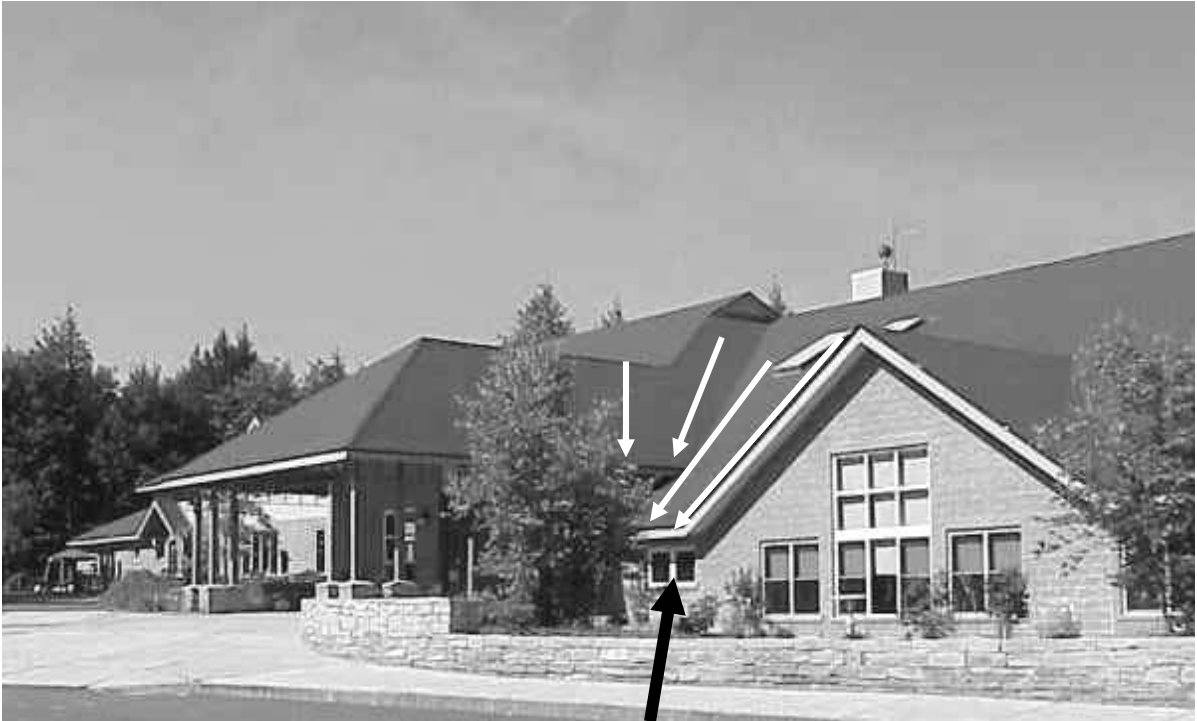
Cafeteria windows with brick cracks
