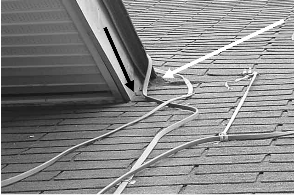
Joint Missing Flashing
