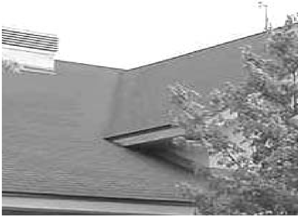
Asphalt Shingled Over Seams, to Create A Cascade Effect of Water Transferring From One Shingle on to Another, Note Lack of Distinct Seam at Roof Tough
