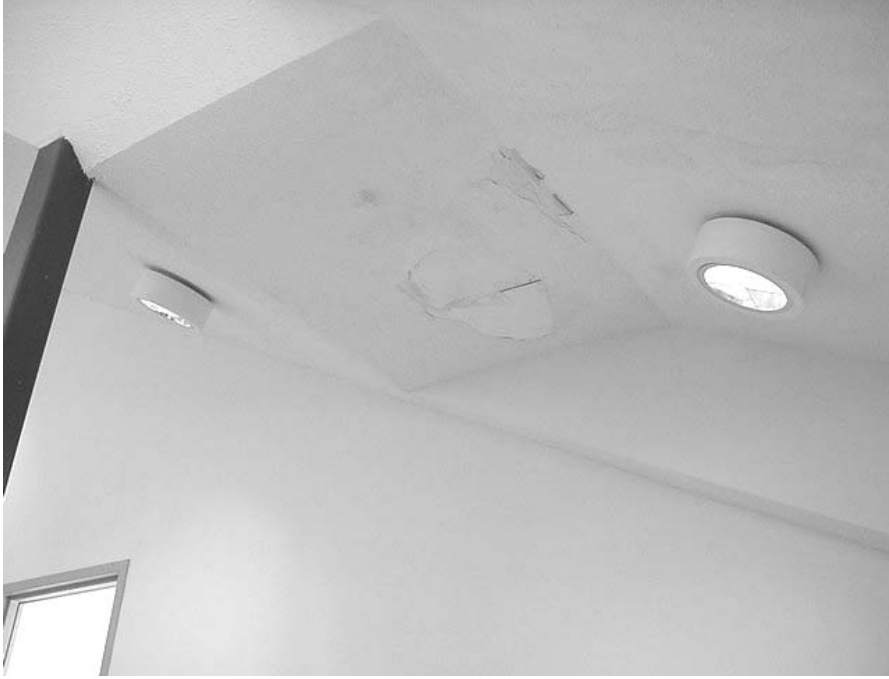
Section of Ceiling That is Chronically Water Damaged
