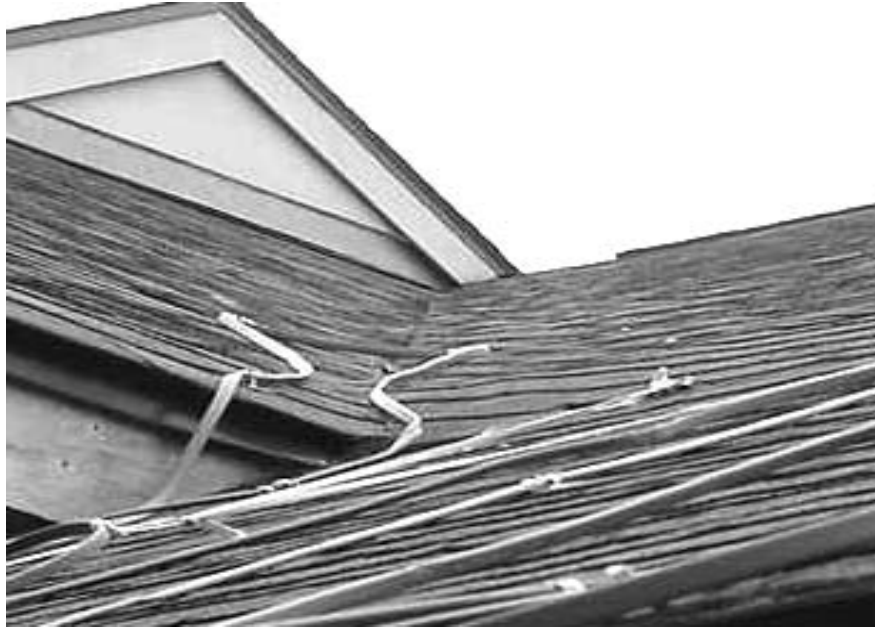
Trough Created by Roof Seam, Note Distinct Seam Created by Shingles Joining at Trough
