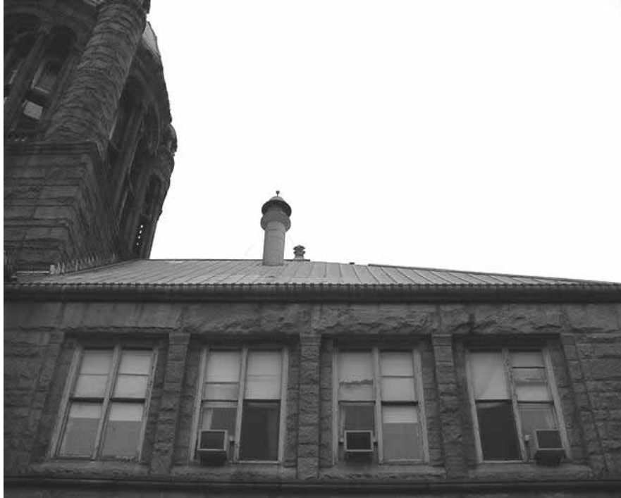
Rooftop Exhaust Vent
