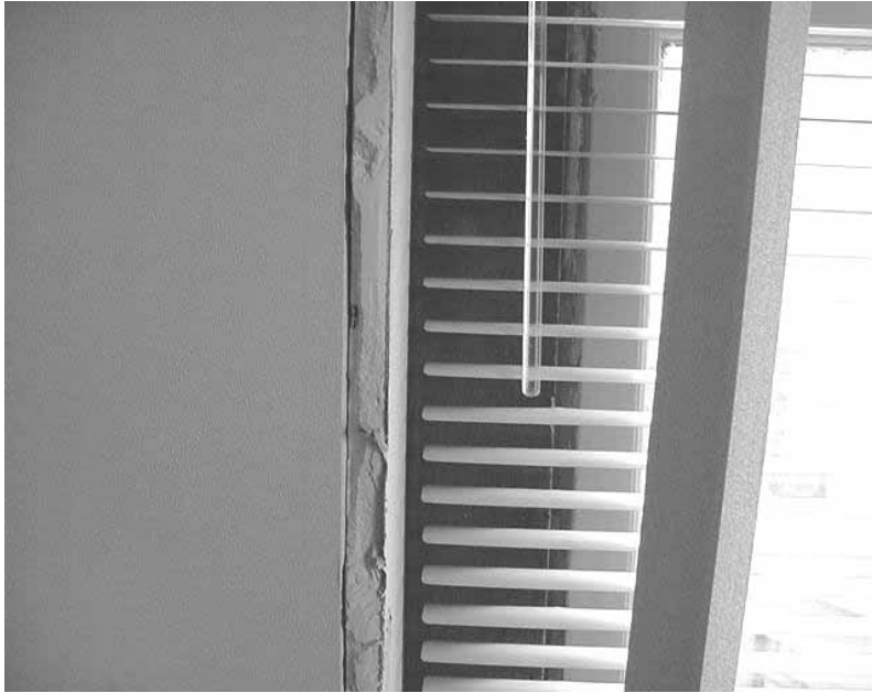
Gypsum Wallboard (GW) Material Was Installed Over the Water Damaged Materials
