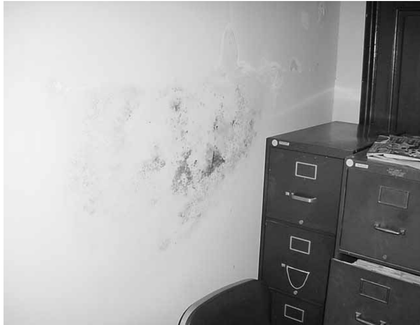
Mold Colonization of Wall behind File Cabinets in Rotunda Balcony
