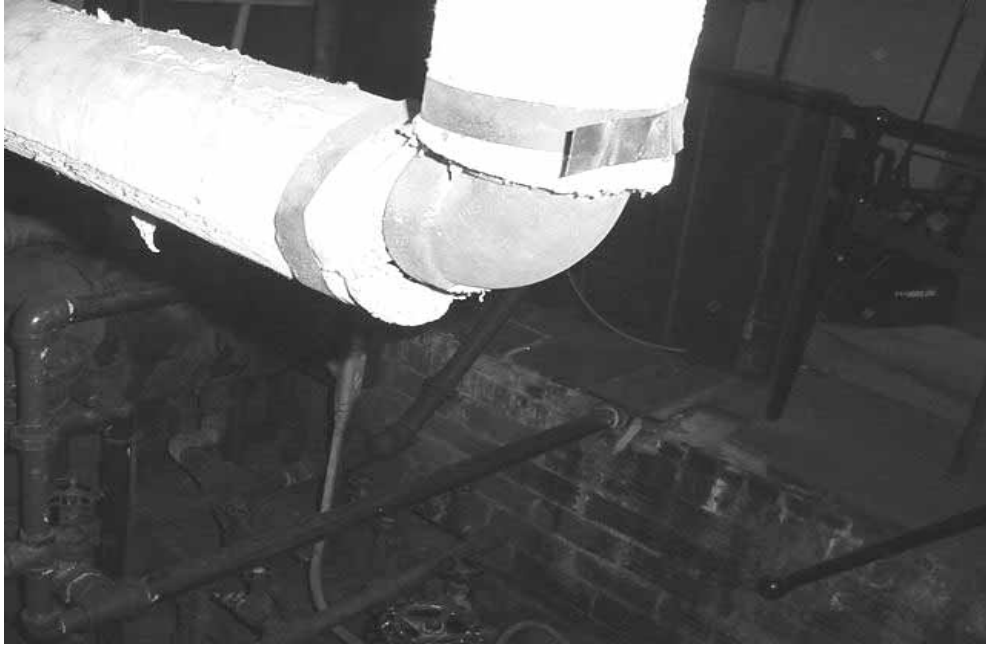
A Pipe Joint with Insulation That Consists Of a White, Powdered Material Was Found In the Basement
