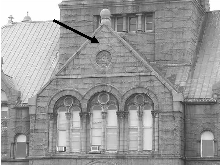
Exterior Façade of BSC Opposite Wall Stains above Clerk's Office Suspended Ceiling
