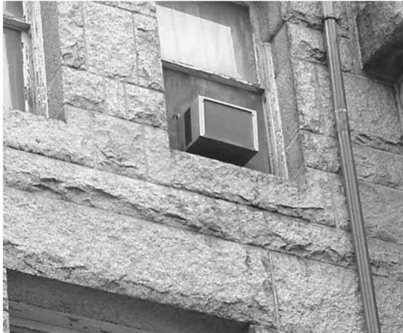
Exterior View of Air-Conditioner Installed In West Facing Wall of Room 62, Note Weathering Of Wood Used To Install the Air Conditioners
