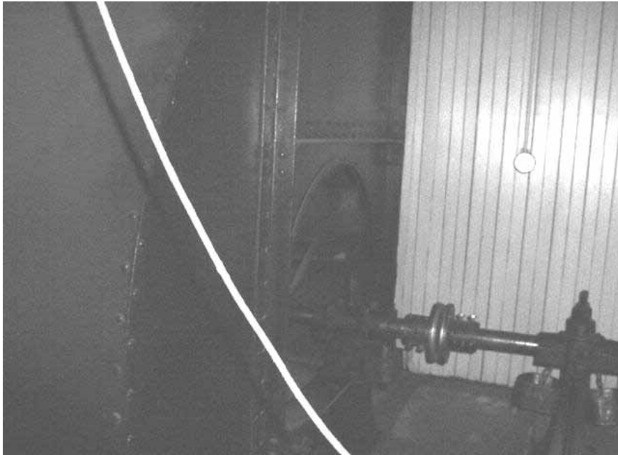
Fresh Air Supply Fan in Basement
