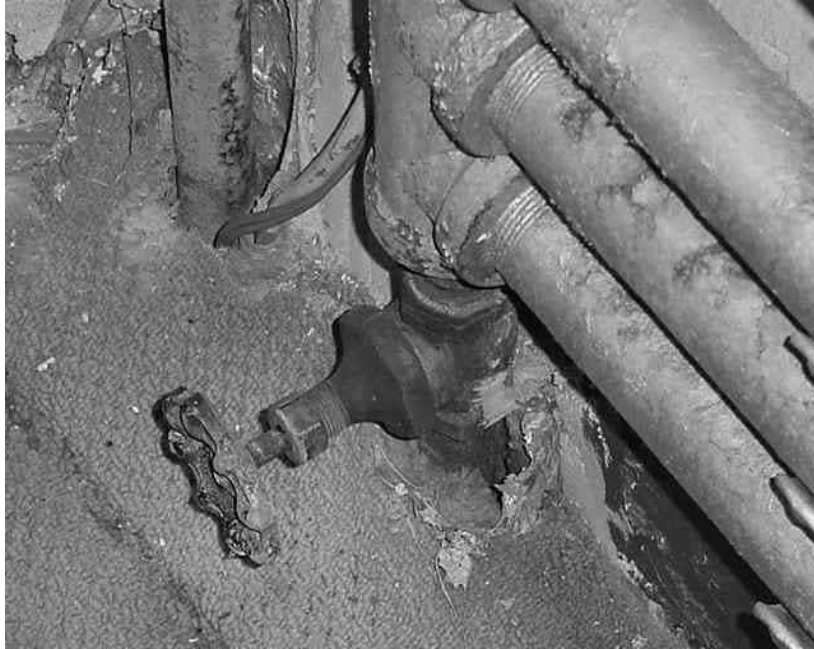
Room 17 Water Damaged Carpet, Likely From Heating System Steam Leak
