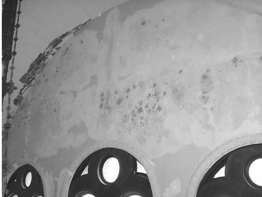
Discoloration of Wall Material above Clerk's Office Suspended Ceiling
