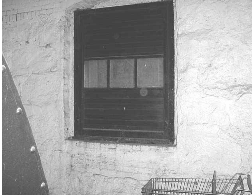
Source of Fresh Air Supply to Basement Fan
