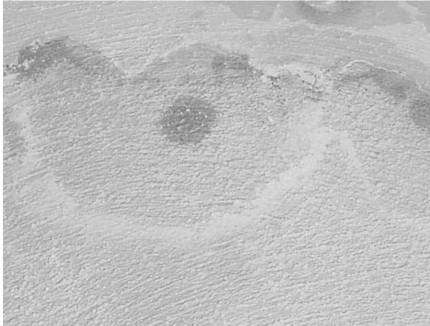
Close-Up of Discoloration of Wall Material above Clerk's Office Suspended Ceiling
