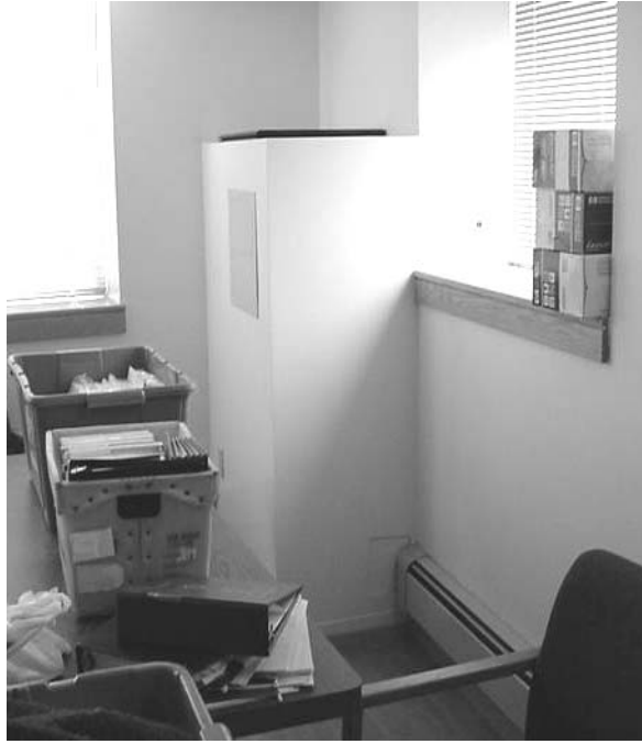
Cabinet Concealing Fire House Standpipe
