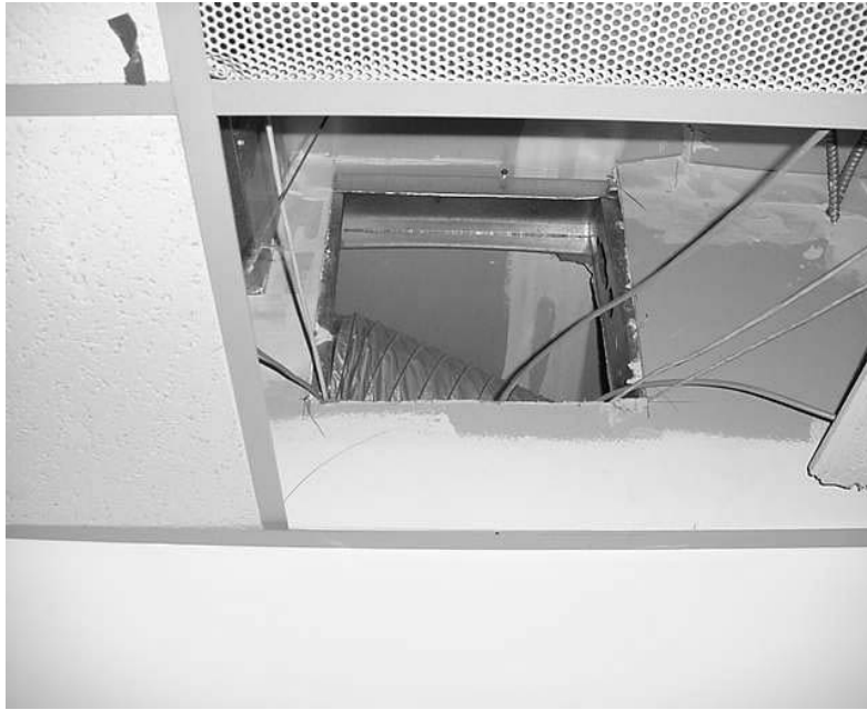
Return Hole For The East Office - 50 Percent Blocked By A Flexible Duct
