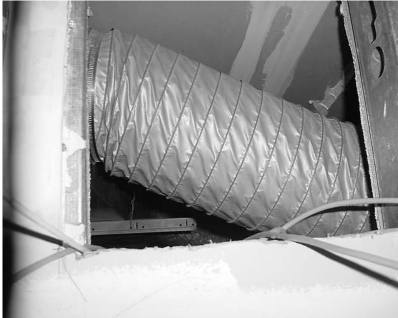
Return Hole For The East Office - 50 Percent Blocked By A Flexible Duct (view at same level as return hole)
