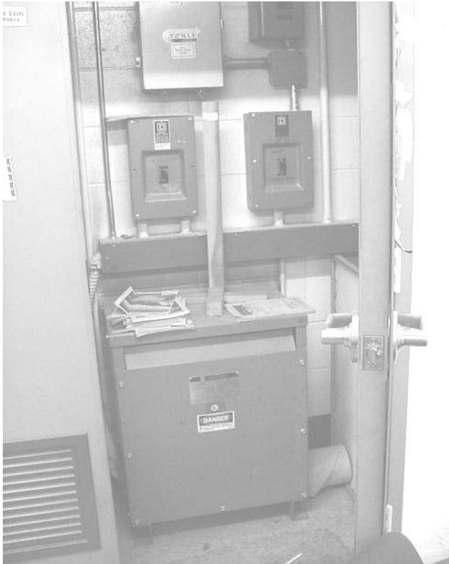
Heat Generating Electrical Equipment in Mechanical Closet in Classroom 120
