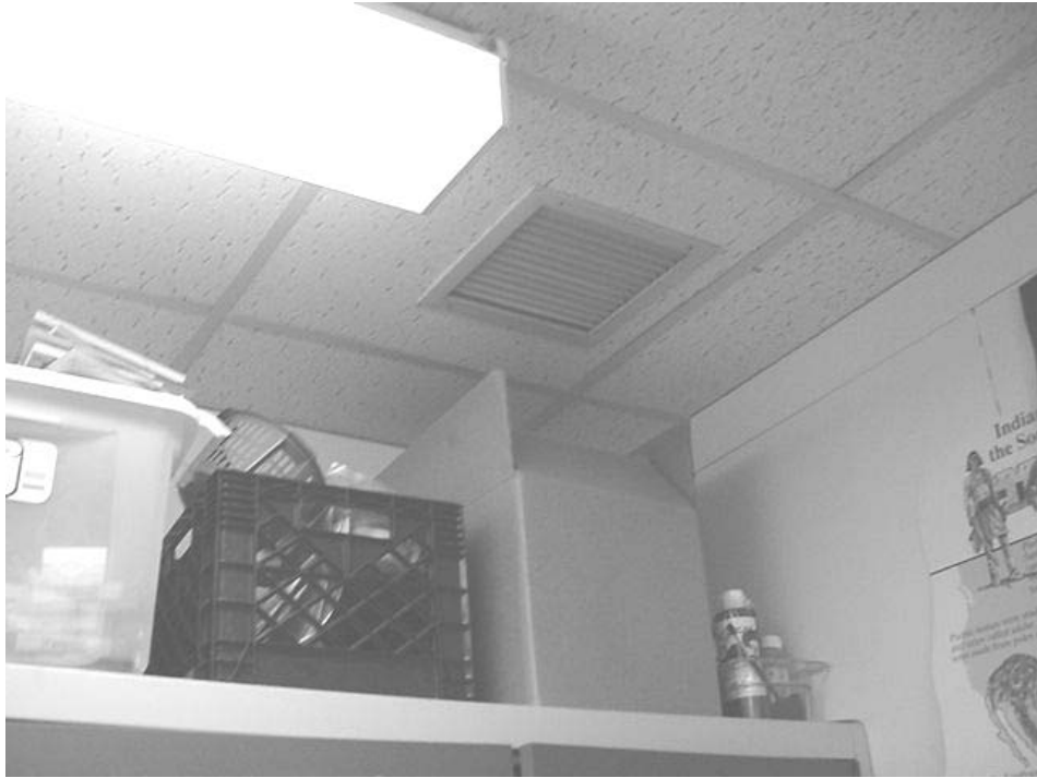
Classroom Exhaust Vent
