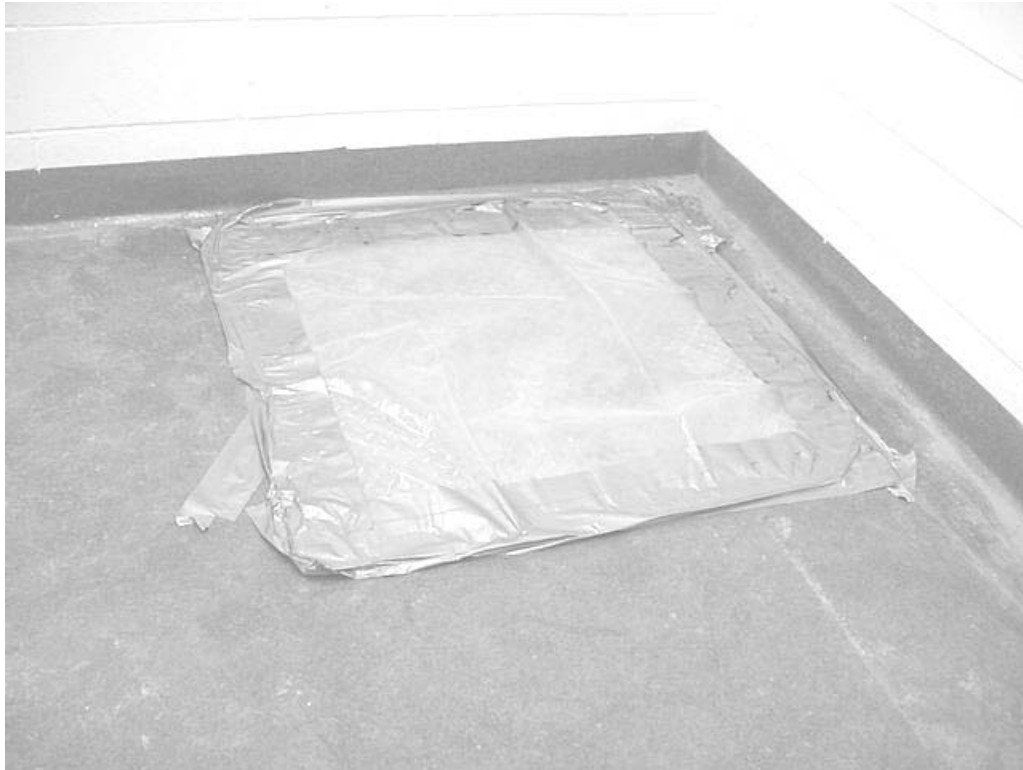
Crawlspace Access Hatch (Room 123) Sealed with Plastic and Duct Tape, Note Crawlspace is Sealed inside as well
