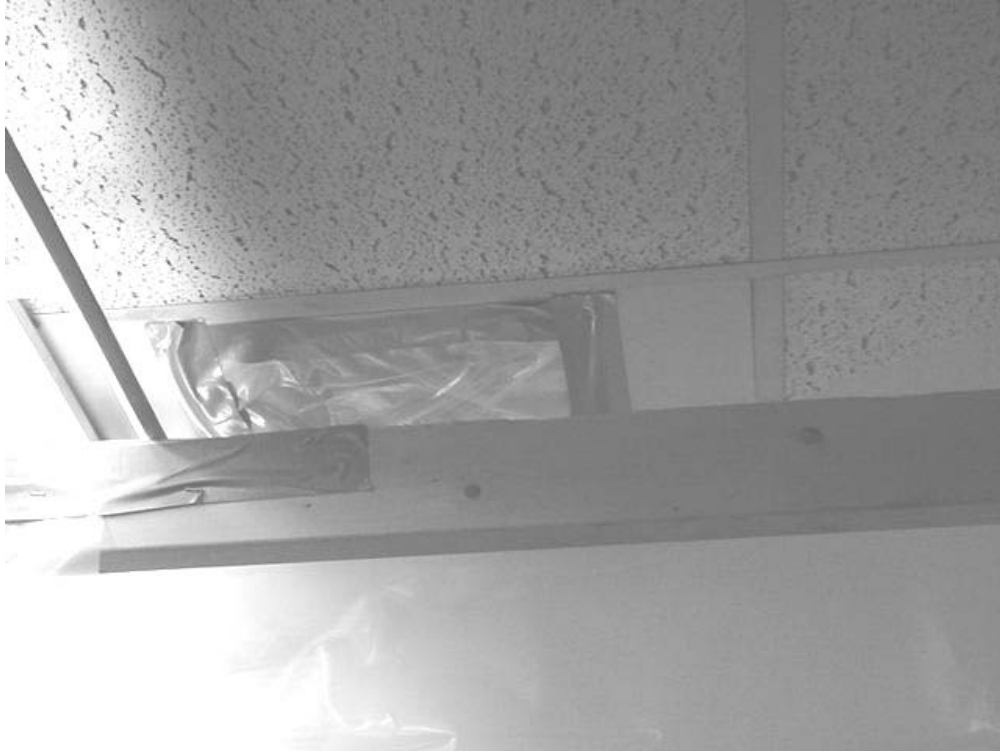
Ceiling Vent Sealed with Plastic and Duct Tape in Classroom 123
