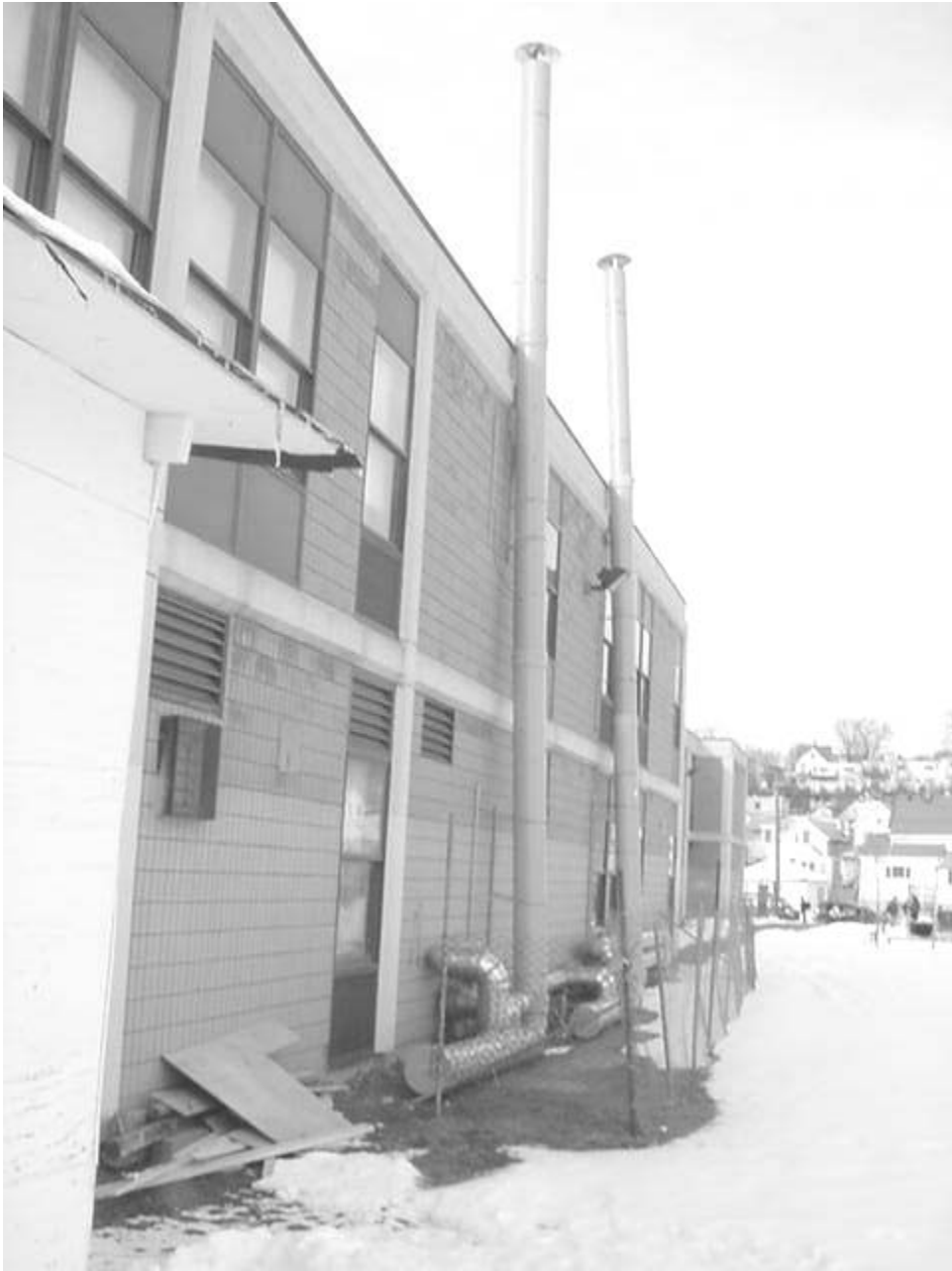
Crawlspace Ventilation System
