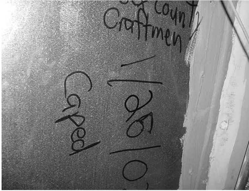
Sheet Metal Installed In Another Duct to Prevent Basement Draw
