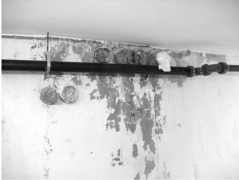
Pipes and Other Holes in the Basement Ceiling Were Sealed With Expanding Foam
