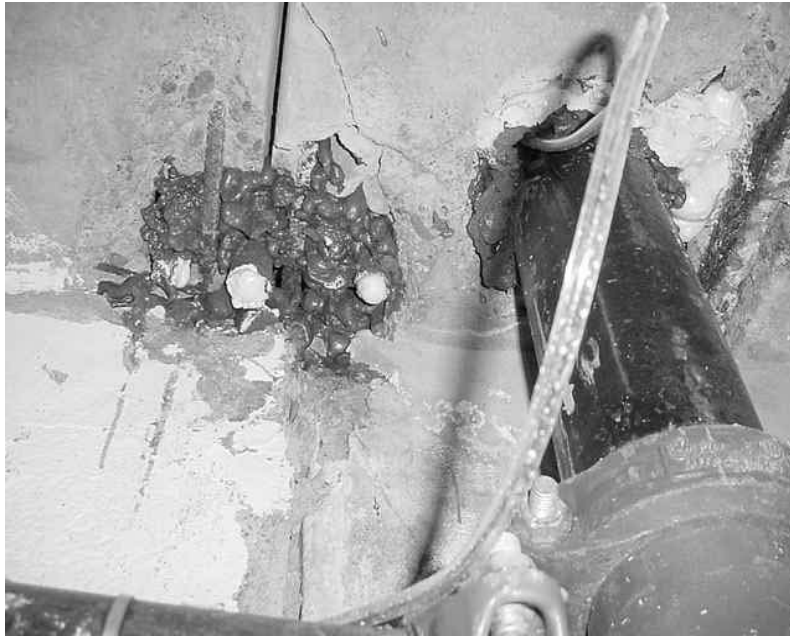
Pipes and Other Holes in the Basement Ceiling Were Sealed With Expanding Foam
