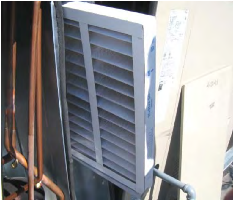
High-Efficiency Pleated Air Filters in Rooftop AHU
