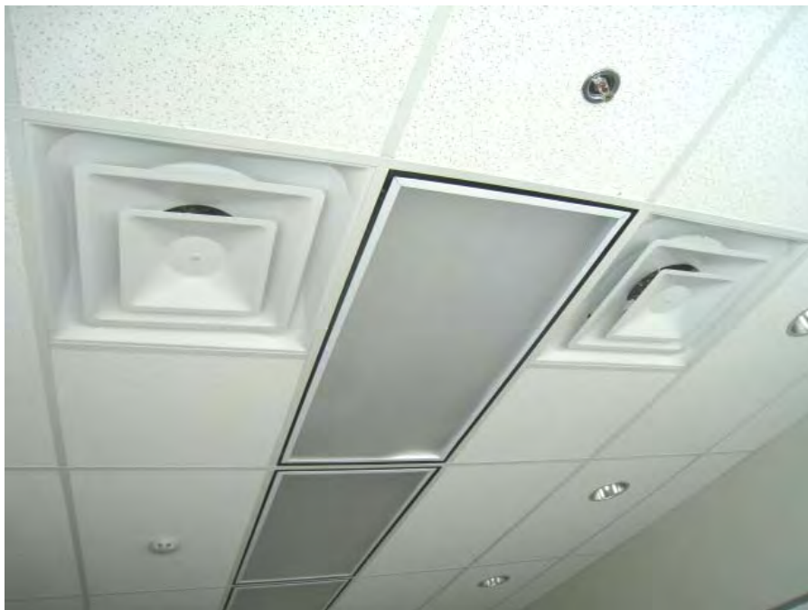
Ceiling-Mounted Supply Diffusers on Left/Right and Slotted Return Vents around Lights
