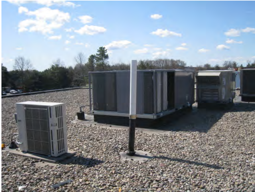
White PVC Vent Stack Extension
