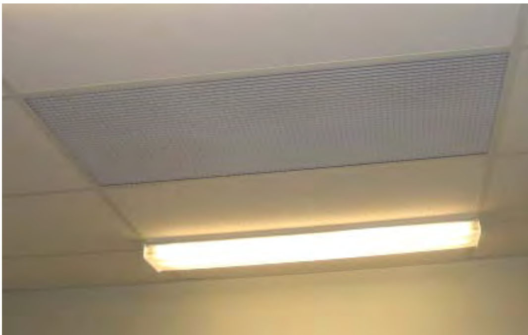
Ceiling-Mounted Return Vent in File Room
