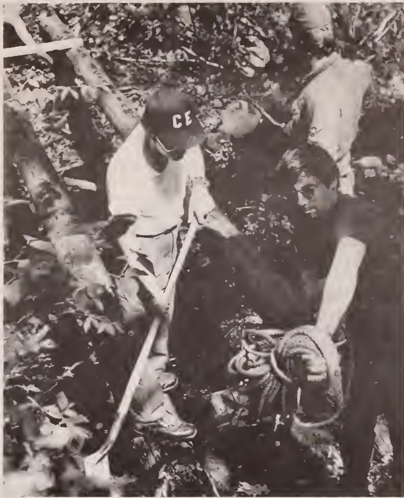
Volunteers from the Westfield Air Guard Civil Engineers are laying telephone poles to make the frame for a foot bridge to be used by children attending the YMCA day camp.
