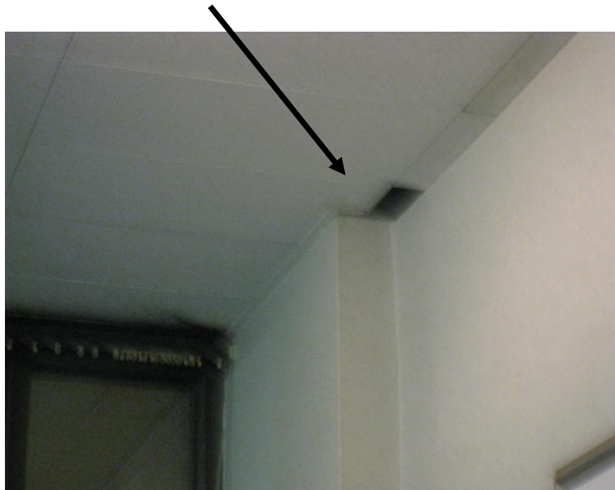
Space in Suspended Ceiling near the Front Desk near Main Entrance to the ROD (arrow)
