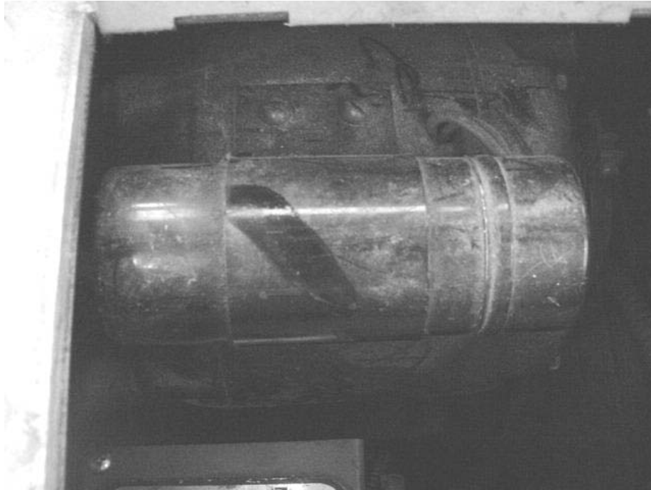
Soot/Dust Accumulation on Motor inside Univent Cabinet
