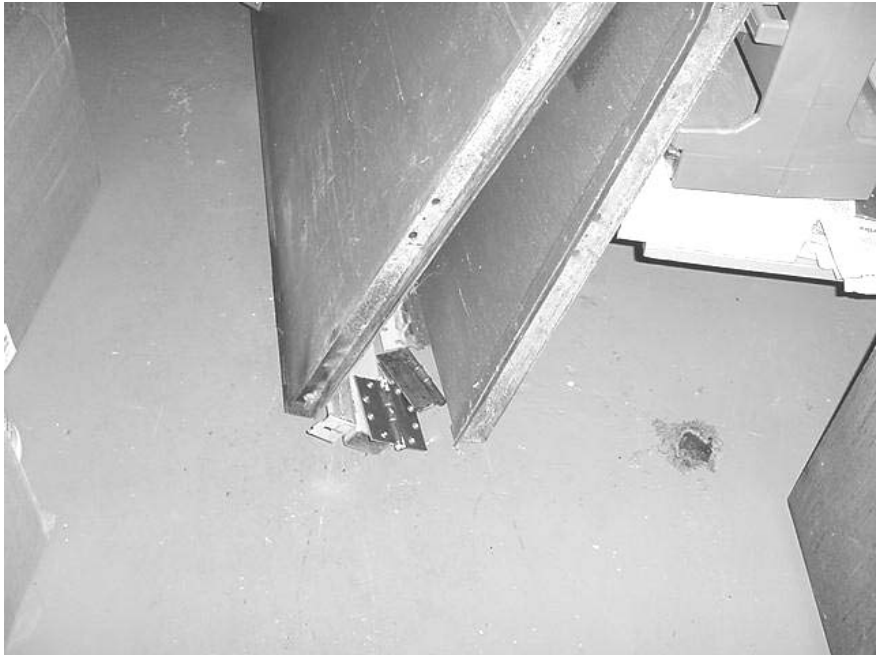
Charred Doors in Art Storeroom
