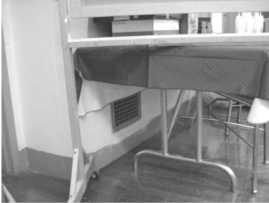
Wall Mounted Exhaust Vent in Art Room, Note Vent is Partially Blocked by Table
