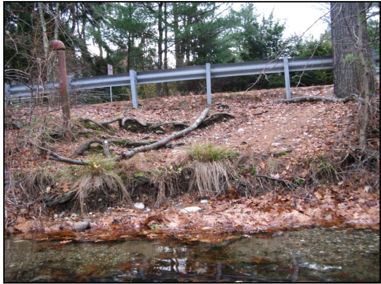
When it rains, storm flow from Federal Street drains directly into Arcadia Lake.
