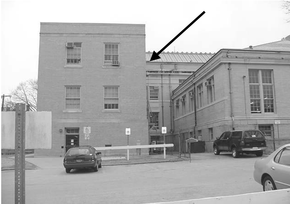
Installation of the New Roof In 1990 Resulted in the Sealing of Original Ventilation Shaft; Arrow Denotes Approximate Location of this Shaft
