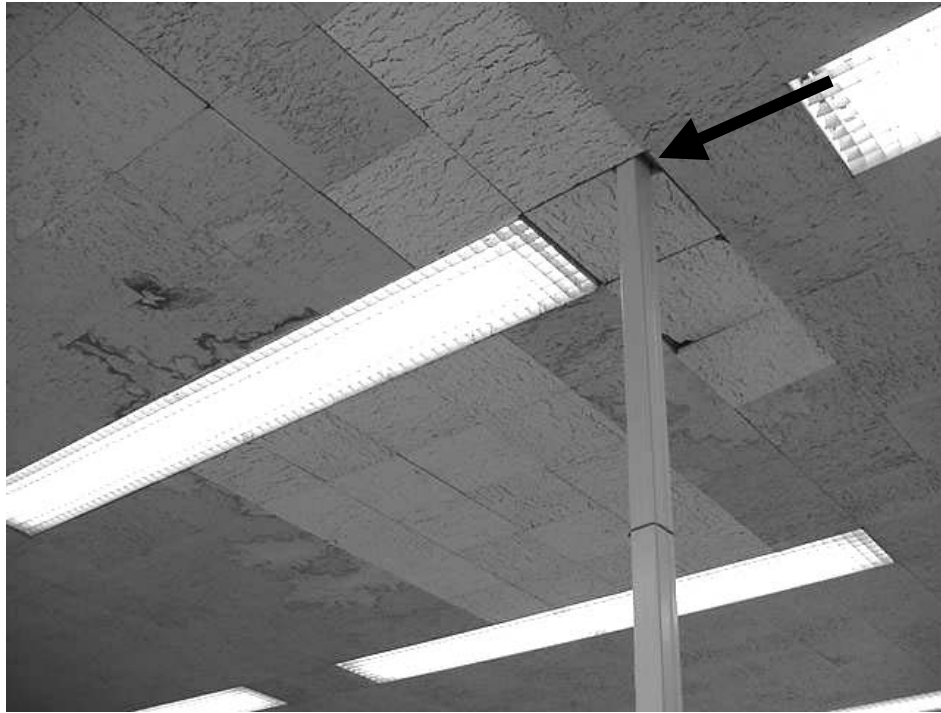
Spaces Continue to Exist in This Ceiling – Family Court Office, 2 nd Floor
