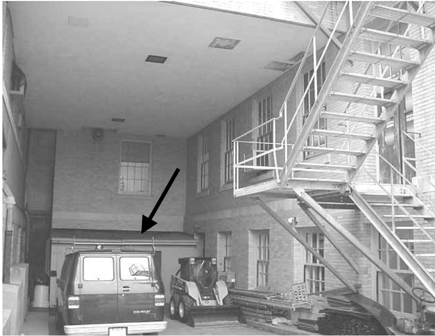
The Fresh Air Intake for the North Mixing Room Was Blocked by the Addition of Storage Sheds During the 1958 Renovations
