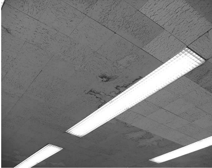
Water-Damaged Ceiling Tiles in the Interlocking System in the Family Court Second Floor South Wing.
