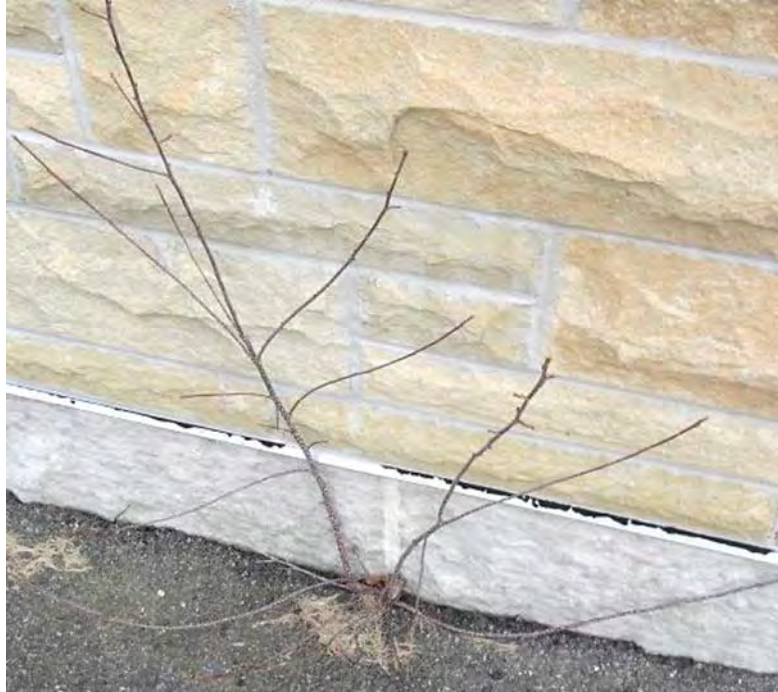
Plant growth against the building foundation
