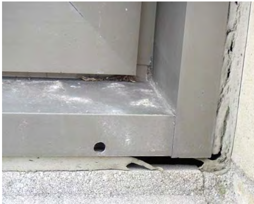
Failing caulking around exterior window
