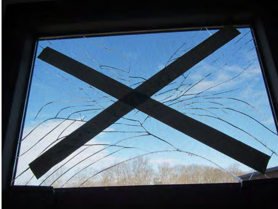
Broken classroom window
