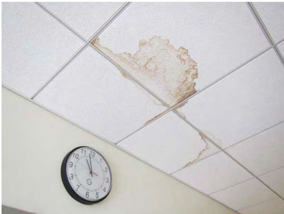
Water-damaged ceiling tiles
