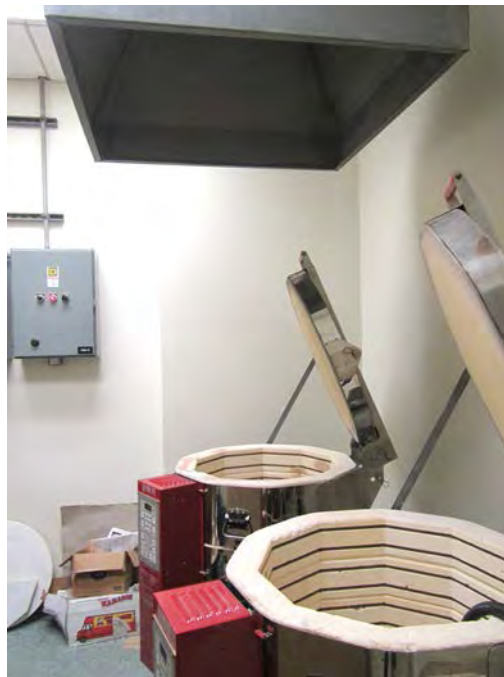
Kiln vent shared between two kilns
