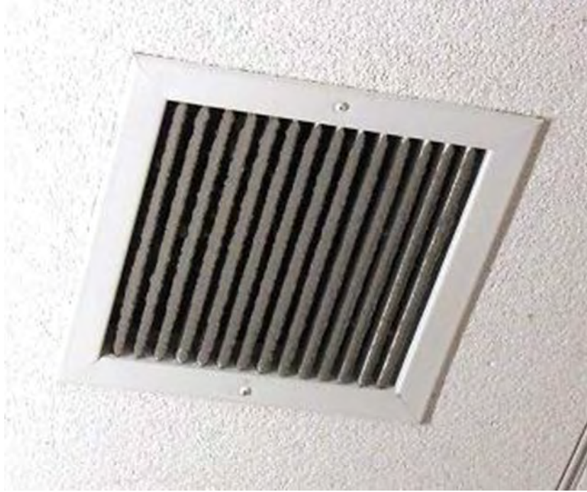
Return grill, note dust/debris accumulation on louvers
