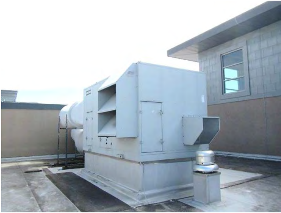
Rooftop air handling unit (AHU)
