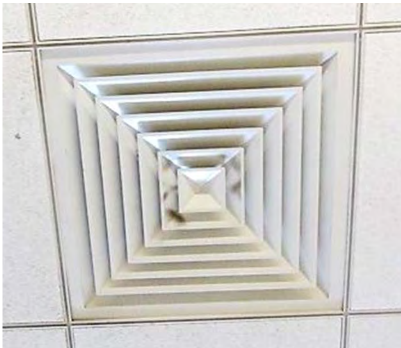
Supply air diffuser, note dust/debris accumulation on louvers
