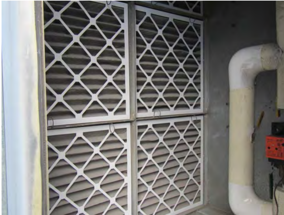
Bank of pleated air filters in AHU
