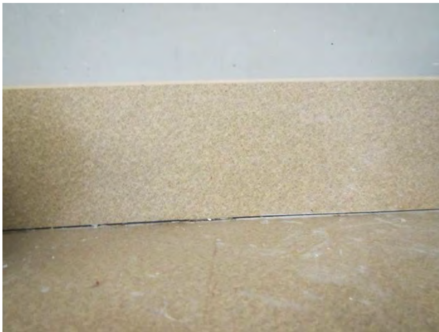
Breach between sink countertop and backsplash
