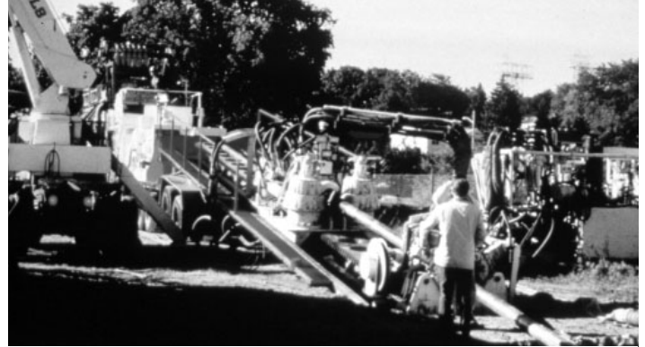
The Horizontal Directional Drilling procedure, shown here at Mill Cove in 1997, begins with the horizontal drilling of an 8-inch diameter pilot hole. The hole is then enlarged until it reaches its ultimate diameter. Finally, the pipeline is pulled through the reamed hole.
