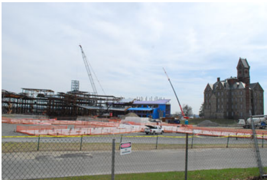
A view of the new facility construction site with the Clock Tower on the right.
