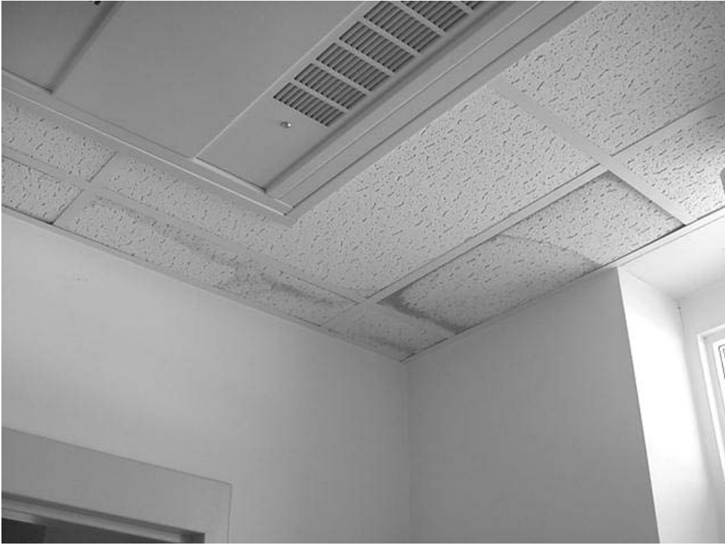
Water Damaged Ceiling Tiles
