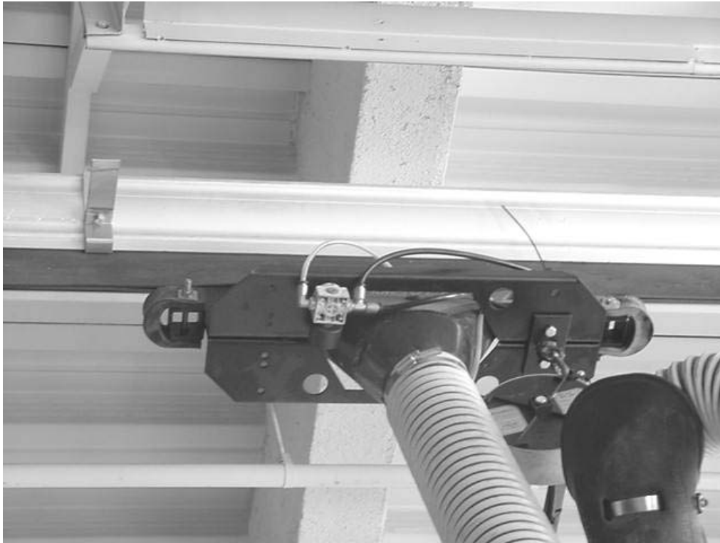
Runner Attached to Flexible Hose for Local Exhaust System in Engine Bay
