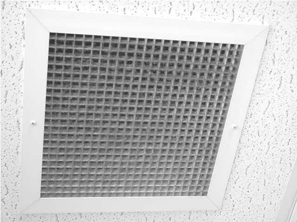
Dirt/Dust Build-up on Return Vent
