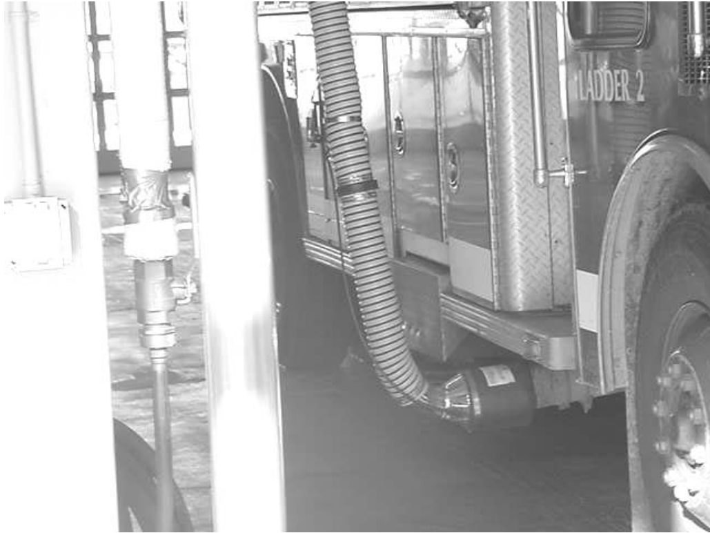
Pressurized Cuff/Flexible Hose for Local Exhaust System in Engine Bay
