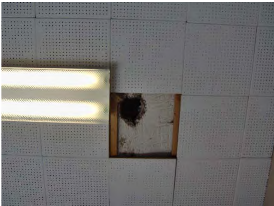
Hole through Ceiling
