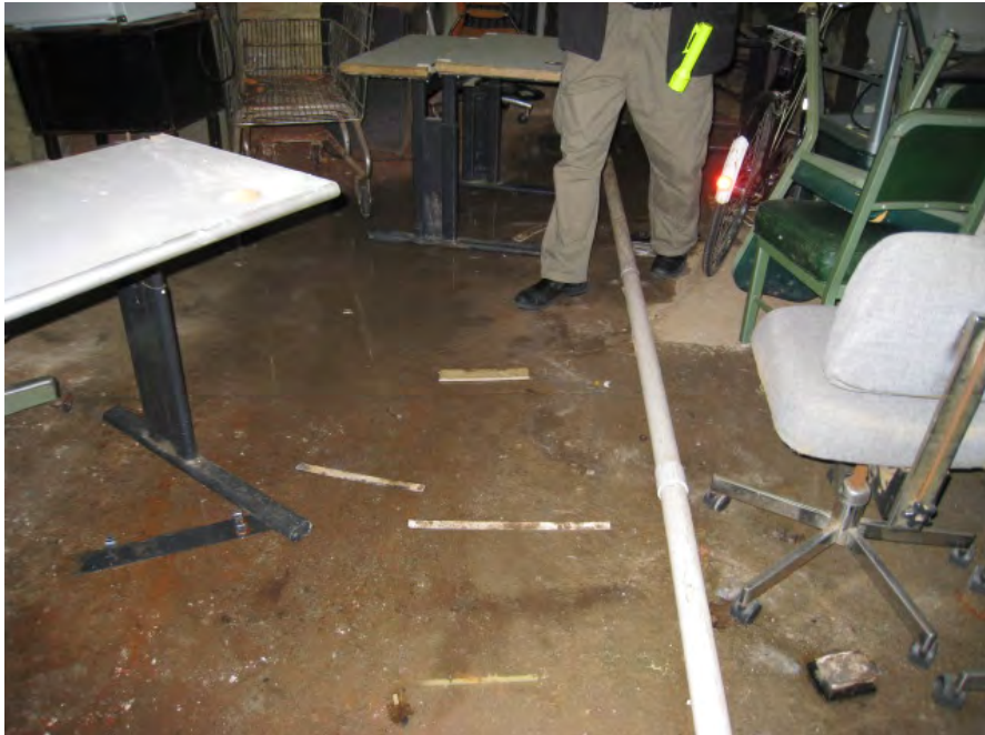
Pipe Connected To Water Collector in Picture 10
