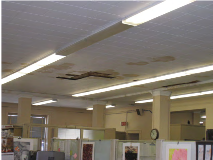
Missing Interlocking Ceiling Tiles
