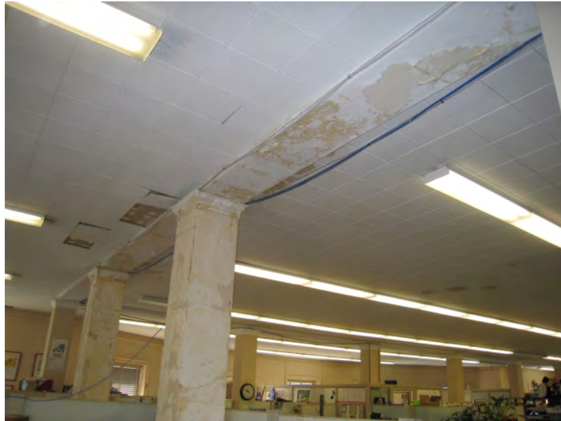
Water Damaged Plaster, 3 rd Floor
