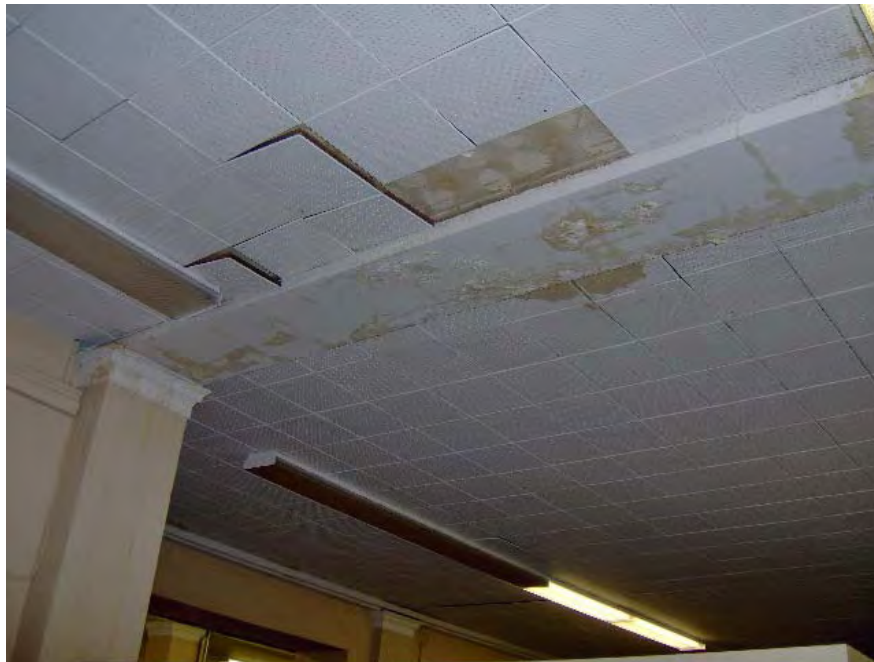
Water Damaged Plaster, 3 rd Floor
