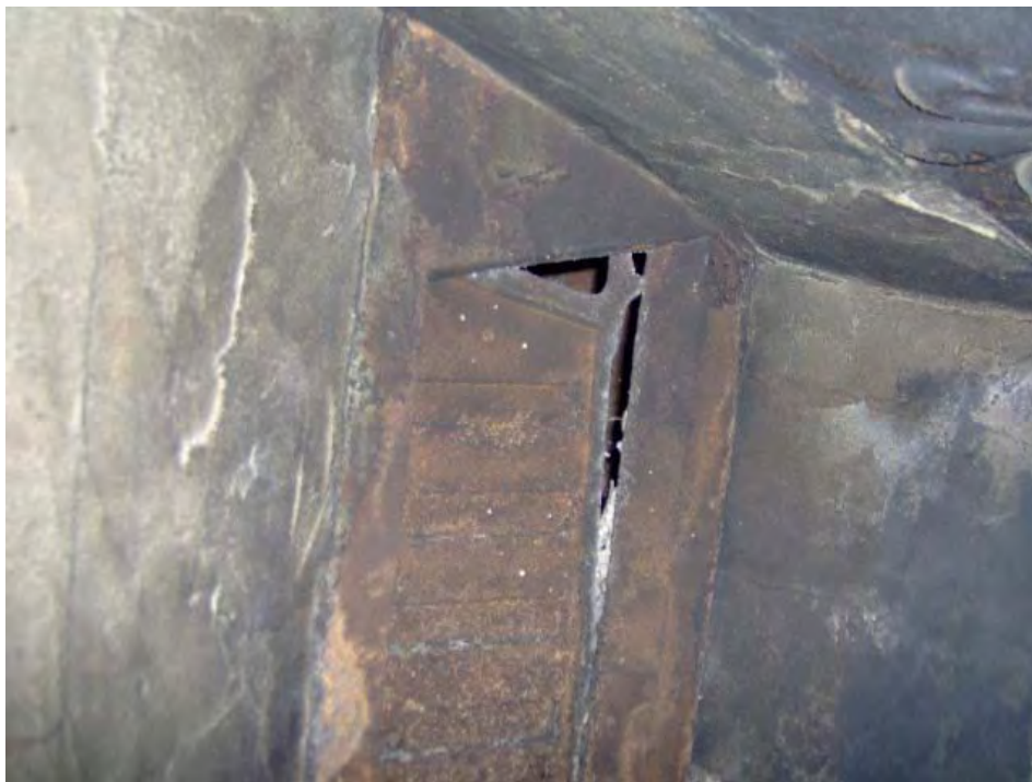
Ajar Flue in Chimney
