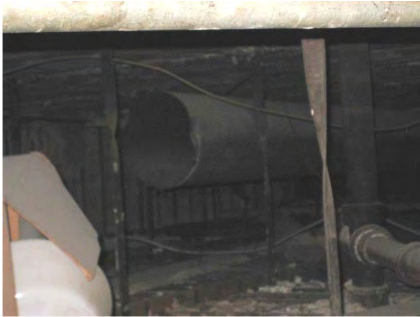
Disconnected Ductwork in Attic
