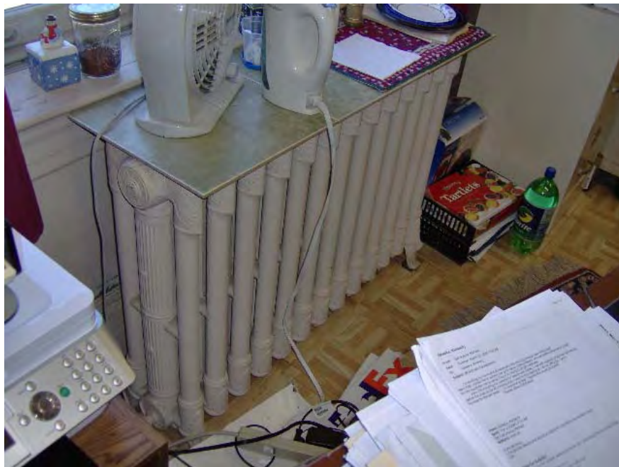
Example of Building Radiator
