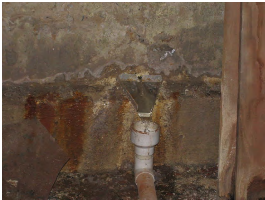
Hole In Foundation Wall Leaking Water, Note Jury Rigged Water Collector
