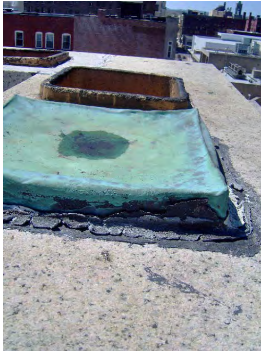
Chimney Openings on Roof, Note Lack Of Chimney Cap
