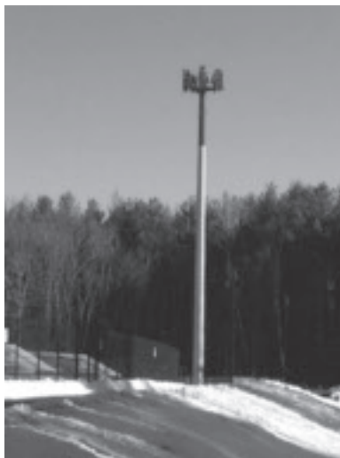
Cell Tower at Glendale Middle Road Landfill
