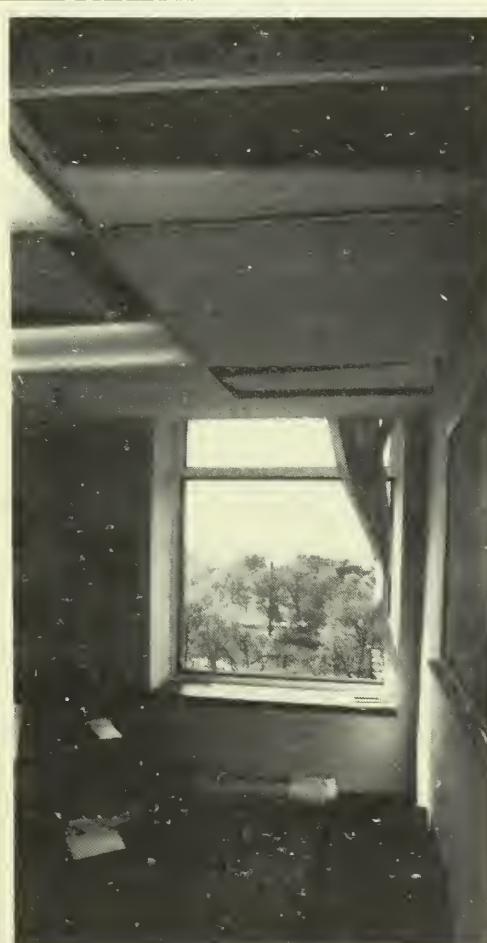
Chief of Staff John Auerbach's office a few weeks ago, shortly after the window was destroyed by high winds. Several staff members were in the office at the time; fortunately, no one was seriously hurt.
