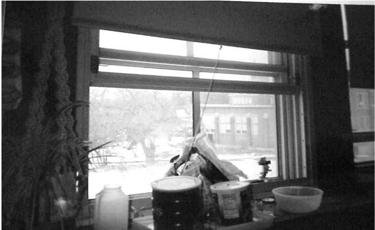
Double-paned Windows Note Inner Window is Opened to Allow for Air Infiltration
