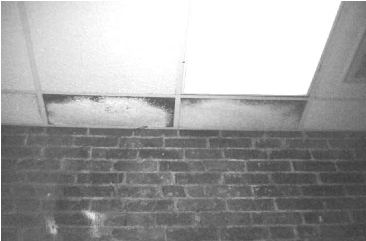
Water-Stained Ceiling Tiles Noted on Third Floor
