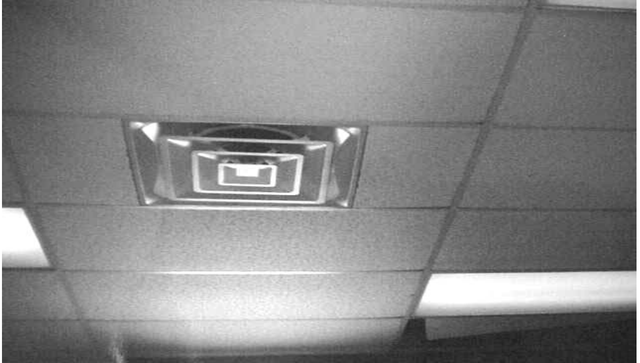
Ceiling-Mounted Air Diffuser Noted on Third Floor
