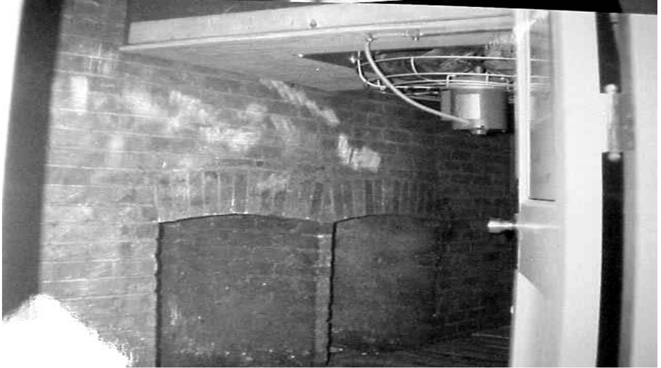
Hearth-like opening for Airshafts in Basement Note Mechanical Fan Installed in Ventilation Shaft
