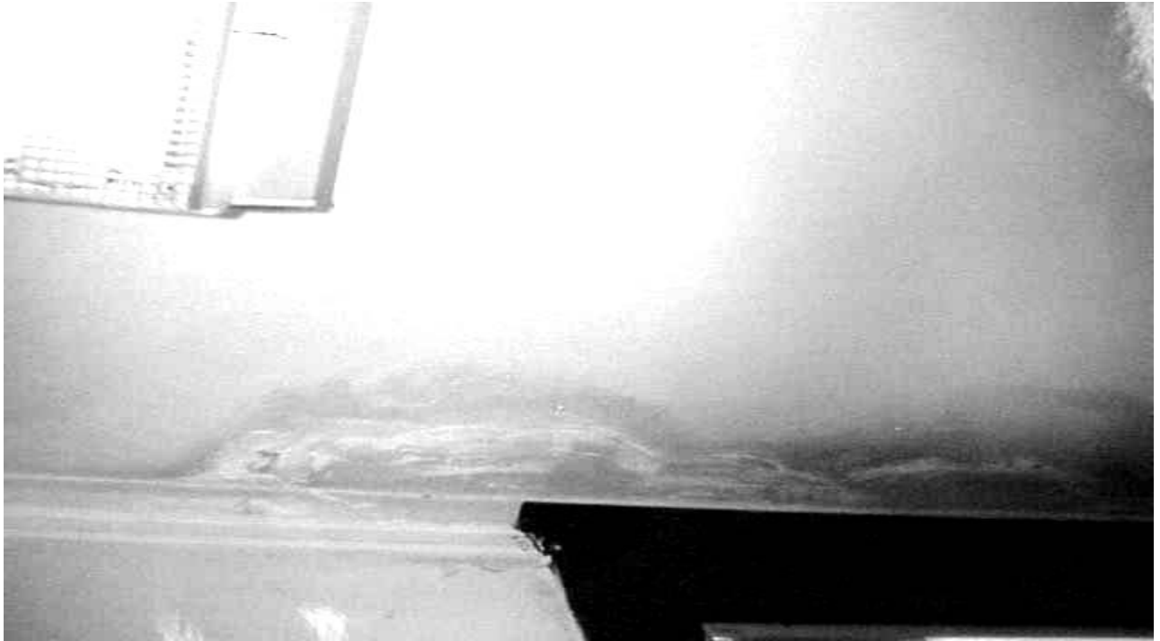
Water-Damaged Ceiling Plaster Noted in Business Office
