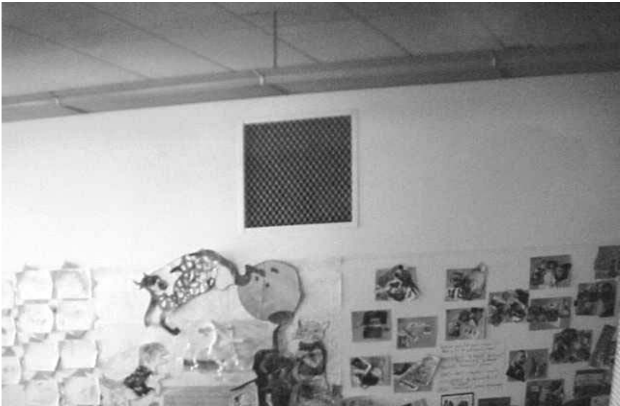
Natural/Gravity Feed Supply Vent in Classroom
