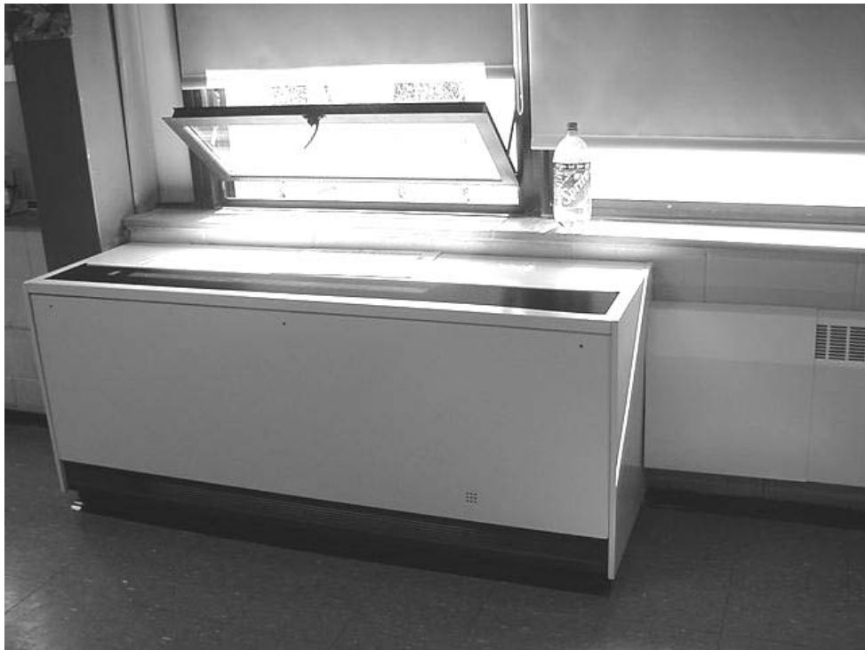
Classroom Univent Note Open Window above Unit
