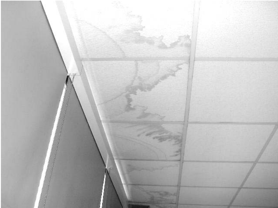
Water Damaged Ceiling Tiles
