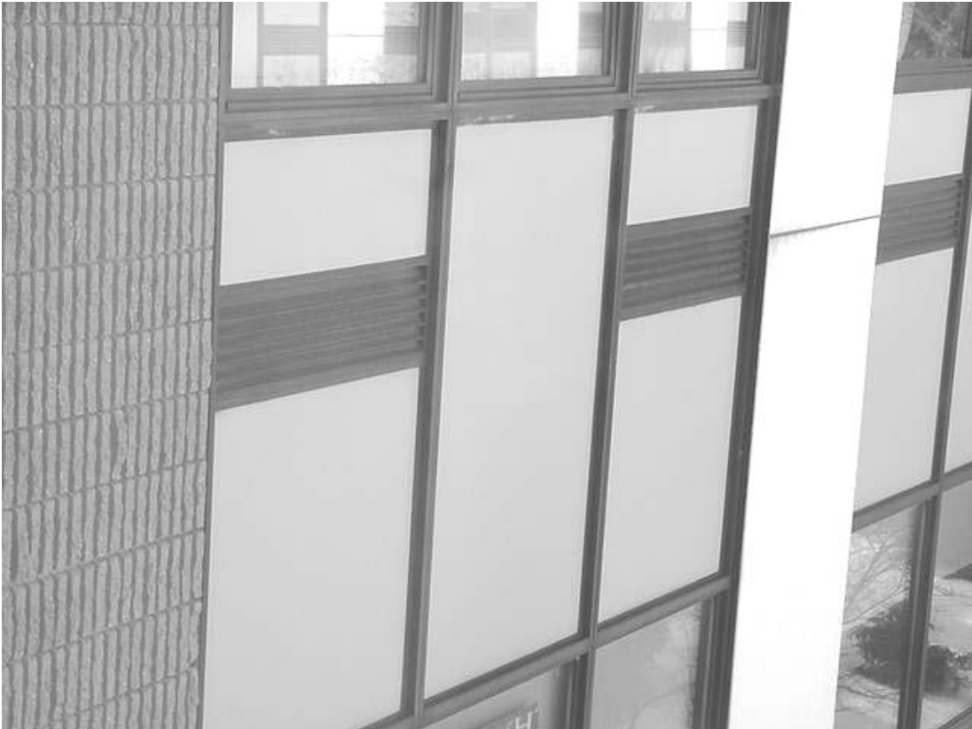
Univent Fresh Air Intakes
