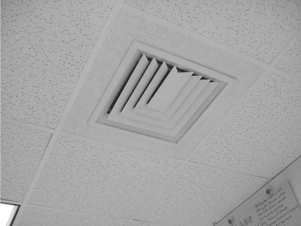
Ceiling-Mounted Return Vent
