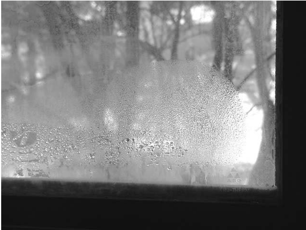
Water Vapor Trapped between Window Panes
