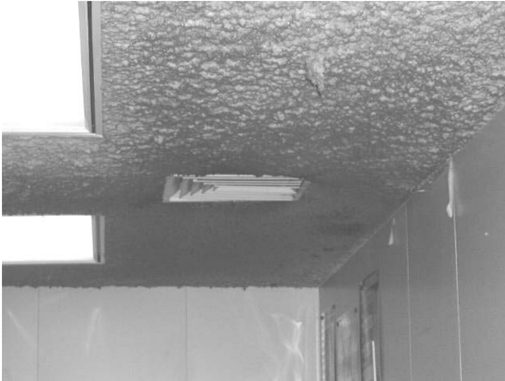
Spray-on Insulation Material Third Floor Ceiling Note Irregular Surface Texture and Staining around Vent
