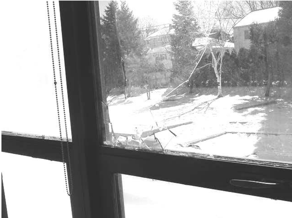
Broken Classroom Window
