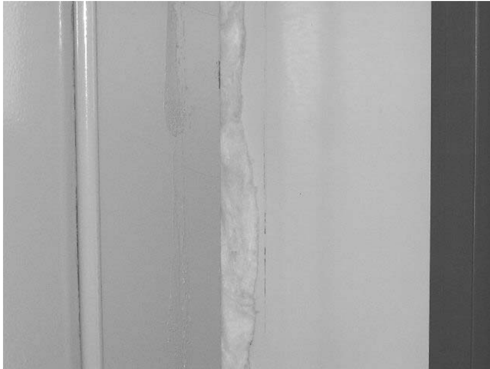
Exposed Fiberglass Insulation in Classroom 231/232
