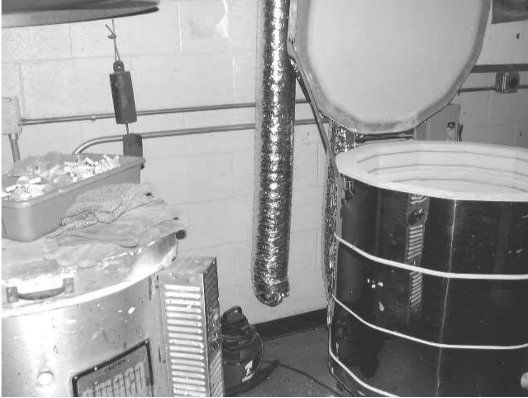
Disconnected Local Kiln Exhaust
