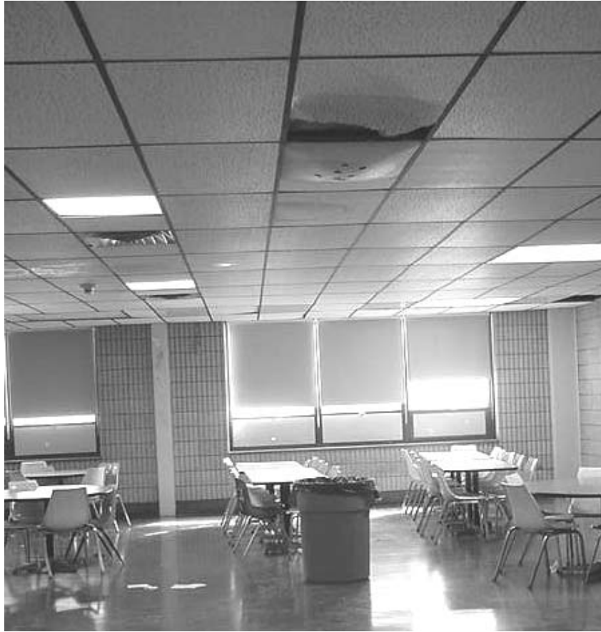
Active Water Leak in Cafeteria Note Garbage Can to Collect Rainwater
