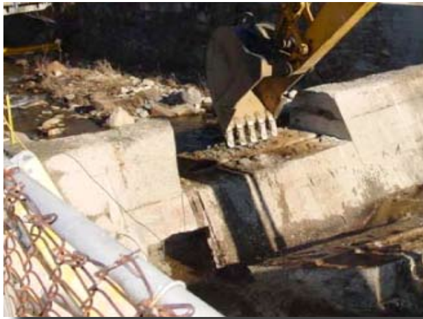
Concrete demolition at the Ballou Dam after a precision dam cut away from the adjacent retaining walls in Becket, MA.
