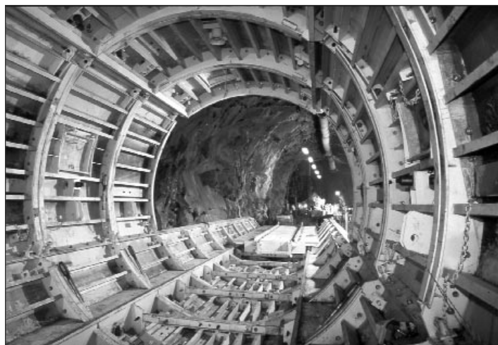
Steel forms positioned around the diameter of the tunnel are ready to receive the concrete mix that forms the tunnel lining.
