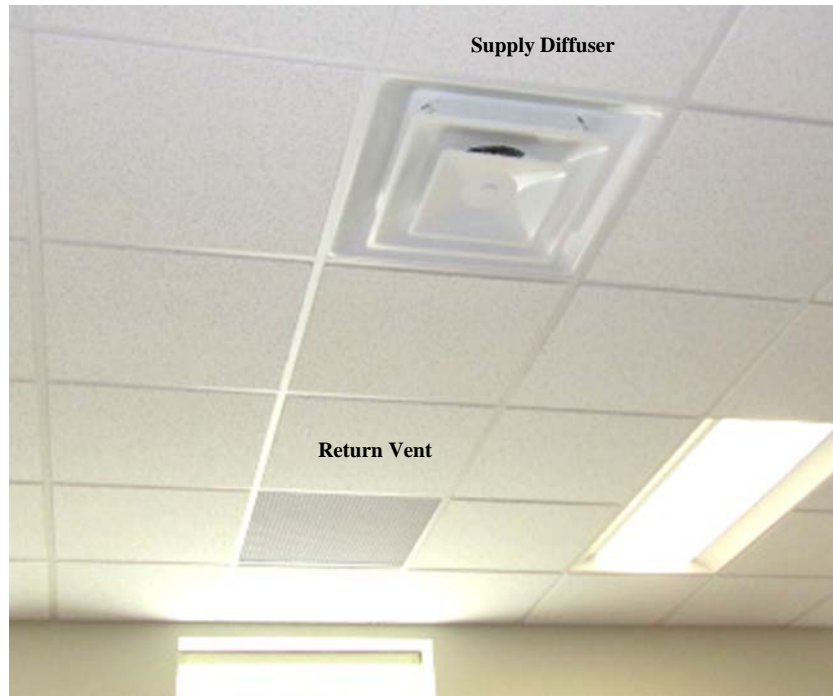
Typical ceiling-mounted supply and return vents
