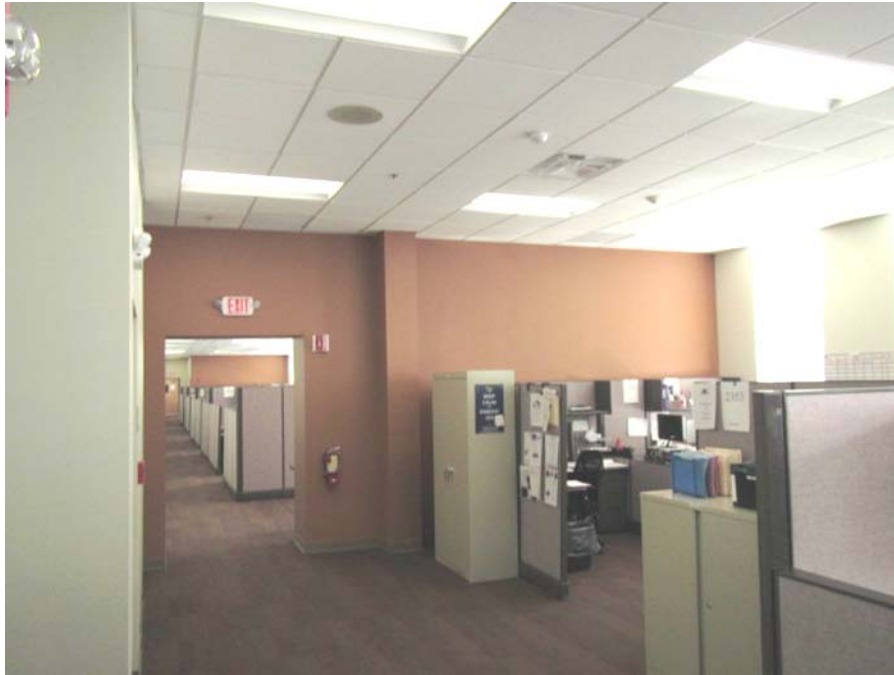
DCF Section 4 where odors were reported/detected
